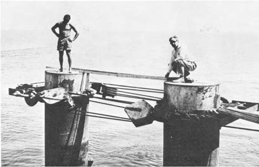
Figure 11.17 Lateral loading test on two steel tubular piles forming part of a breasting dolphin.
