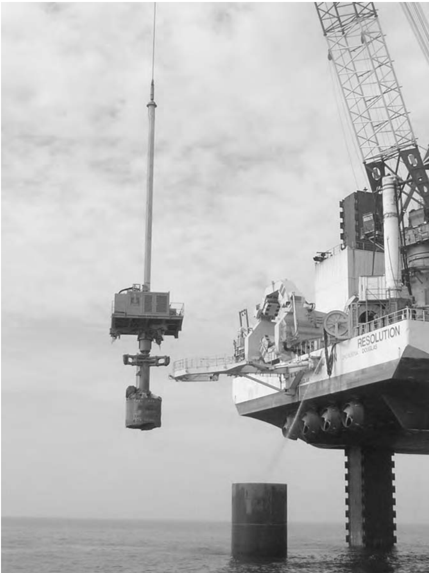
Figure 3.27 'Flydrill 5500' with bucket auger removing spoil from 4.75 m dia monopiles at the Barrow offshore wind farm site (courtesy Bauer Maschinen GmbH).
