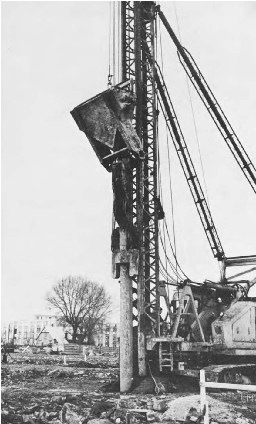
Figure 3.24 Discharging concrete into the driving tube of a withdrawable tube pile. Concreting skip travelling on pile frame leaders.
