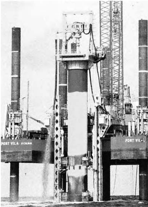
Figure 3.7 Installing a 4 m dia monopile foundation for North Hoyle offshore wind farm with pile top rig and specially designed leader leg pile frame (courtesy Seacore Ltd).
