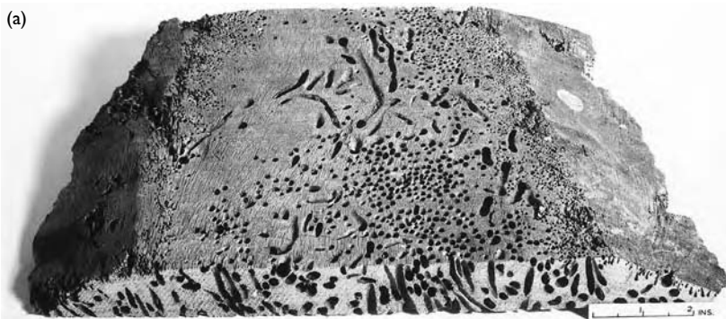
Figure 10.2 Attack on timber piles by marine borers (Crown copyright reproduced with permission of BRE) (a) Attack by Teredo (b) Attack by limnoria .
