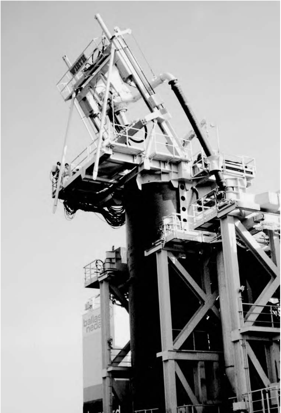
Figure 9.23 Drilling equipment for sinking 3.5 m OD precast concrete cylinder piles, Saudi Arabia–Bahrain Causeway.
