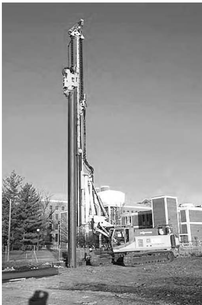
Figure 3.1 ABI Mobilram with telescopic leader fully extended driving tubular pile (courtesy ABI GmbH).
