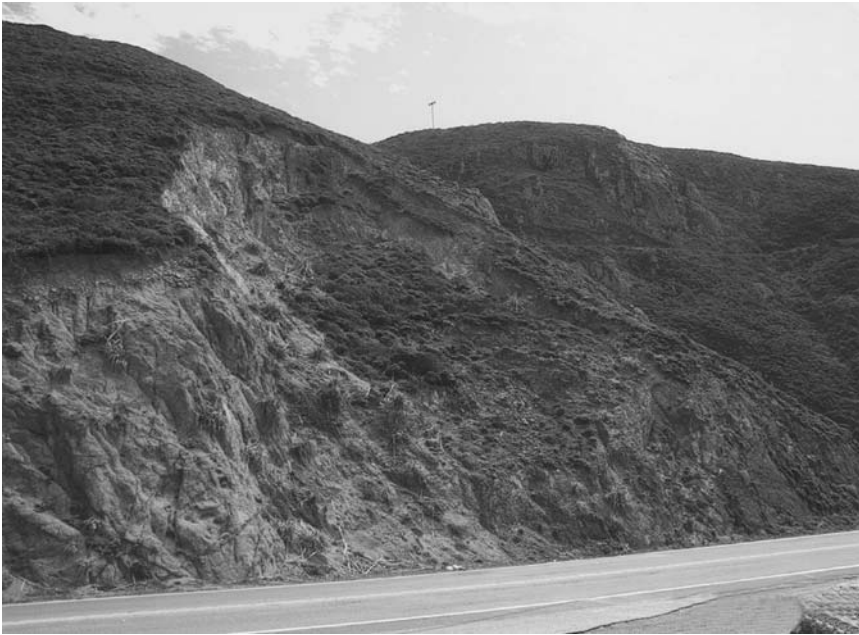
Figure 8.1 Circular failure in highly weathered, granitic rock (on Highway 1, near Devil's Slide, Pacifica, California).
