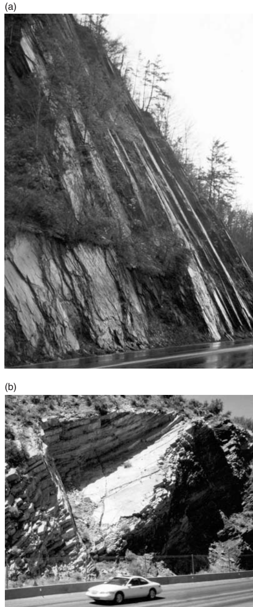
Figure 2.1 Rock faces formed by persistent discontinuities: (a) plane failure formed by bedding planes parallel to face with continuous lengths over the full height of the slope (shale on Route 19 near Robbinsville, North Carolina); (b) wedge failure formed by two intersecting planes dipping out of the face (sedimentary formation on Route 60 near Phoenix, Arizona).
