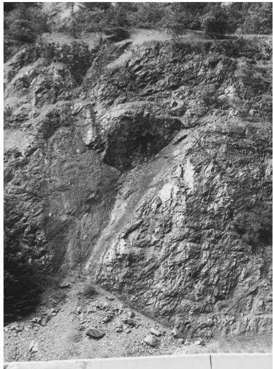
Figure 7.1 Typical wedge failure involving sliding on two persistent joints with line of intersection of joints daylighting at toe of rock face, and an upper plane that formed a tension crack (strong, volcanic rock on Interstate 5, near Grants Pass, Oregon).
