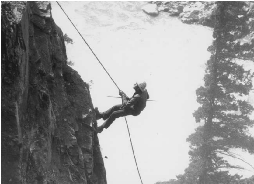
Figure 12.18 High scaler suspended on rope and belt while removing loose rock on steep rock slope (Thompson River Canyon, British Columbia, Canada) (TRB, 1996).
