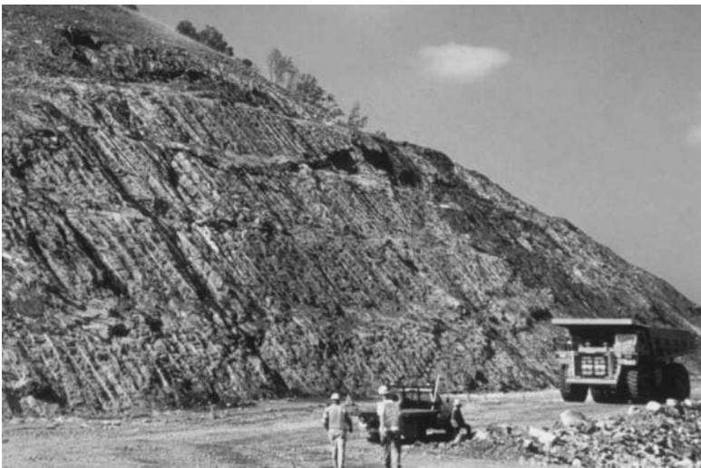
Figure 11.10 Example of controlled blasting for rock cut on highway project (strong, highly folded gneiss, I-26/US23, near Mars Hill, North Carolina) (courtesy: North Carolina Department of Transportation).
