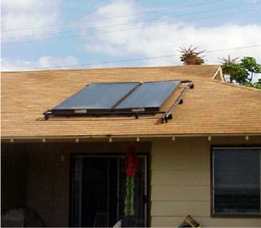
Figure 1.7 Flat-plate thermal solar collectors for providing hot water.(photo courtesy of DOE/NREL, Warren Gretz)
