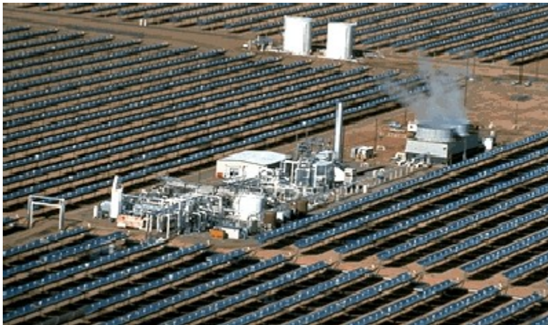
Figure 1.12 One of the steam cycle power cycles at the Kramer Junction solar energy generating system.(photo courtesy of DOE/NREL, Warren Gretz)
