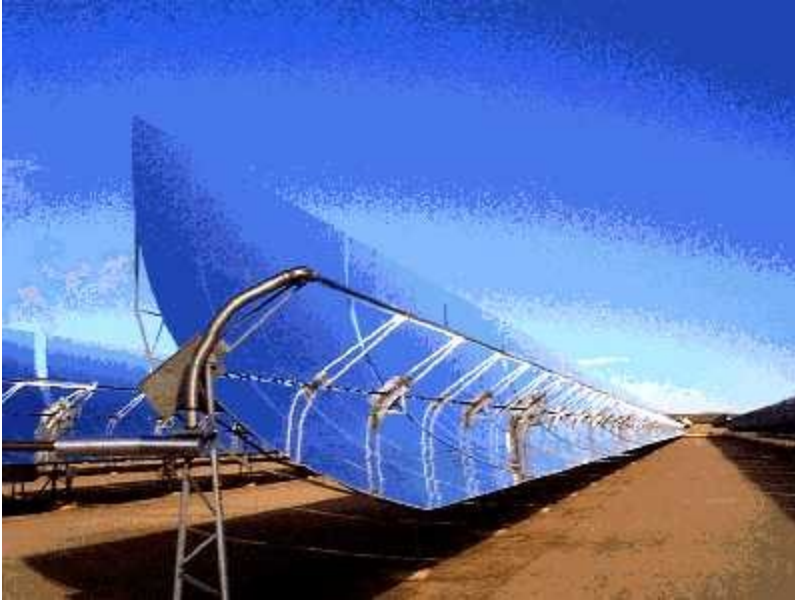
Figure 1.10c A single-axis tracking parabolic trough collector. (courtesy of Kramer Junction Operating Company)
