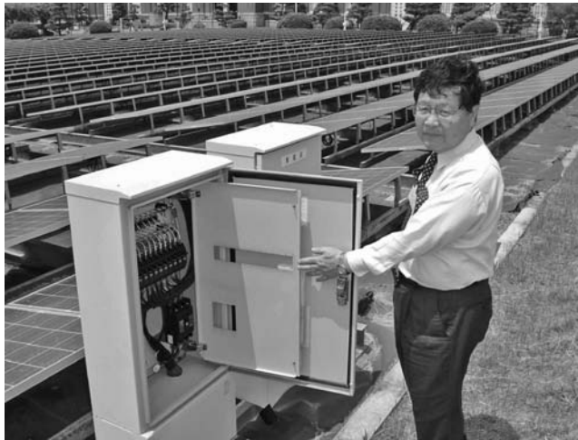
FIGURE 8.5 Project designer Mr. Ohashi and Osaka Waterworks Kunijima Treatment Plant with a 150 kW p PV plant (Kyocera), one of over a dozen such PV water plants in Japan.
