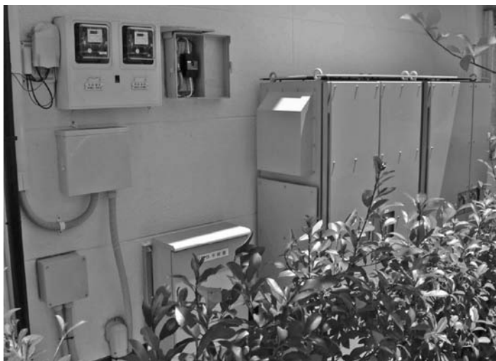
FIGURE 8.6 PV system grid inter-tie (note 2 meters) in Ohta City. Inverter and battery bank are housed in the large boxes on the right.
