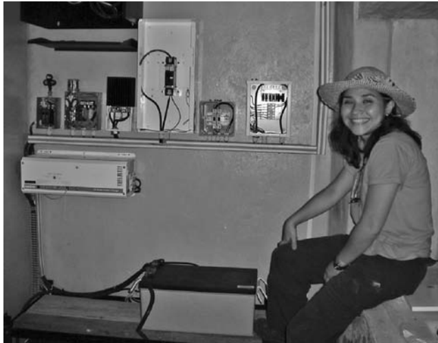
FIGURE 8.22 PV-powered COHCIT satellite telecenter with Internet connectivity using quality BOS components with master PV installer Ethel Enamorado in Sosoal, Lempira, Honduras.
