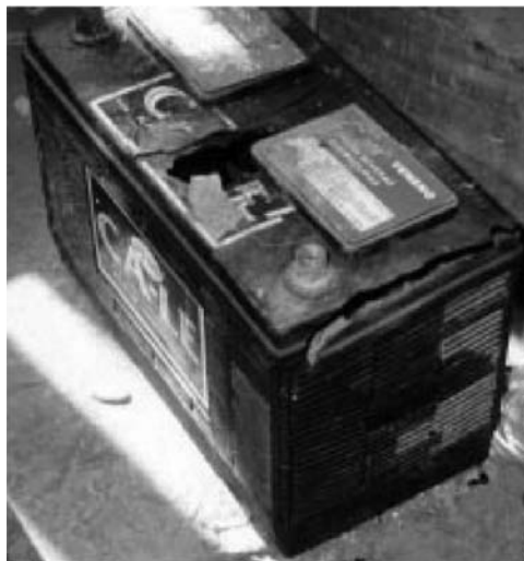
FIGURE 11.14 Exploded battery at Chiapas residence from ungrounded PV system hit by lightning.
