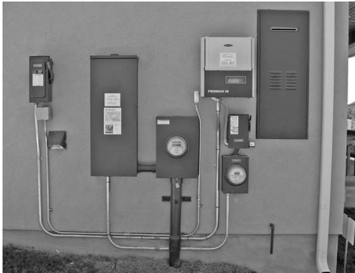
FIGURE 6.14 Utility interactive PV system installation in Austin, Texas (2008). Note the DC and AC disconnects, electric meters, and Fronius inverter.
