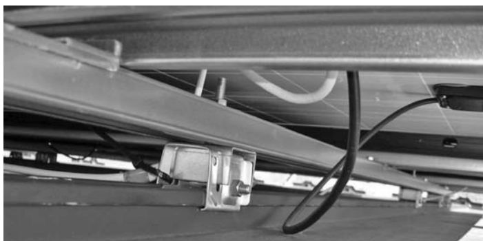
FIGURE 8.8 Underside of typical Japanese PV array clamp mounting on metal corrugated roof (no roof penetration) designed to withstand typhoon force winds.
