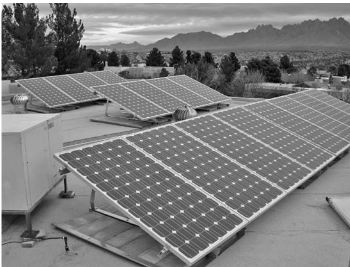
FIGURE 6.8 PV modules tilted to maximize annual energy production for utility interactive residential installation in Las Cruces, New Mexico.
