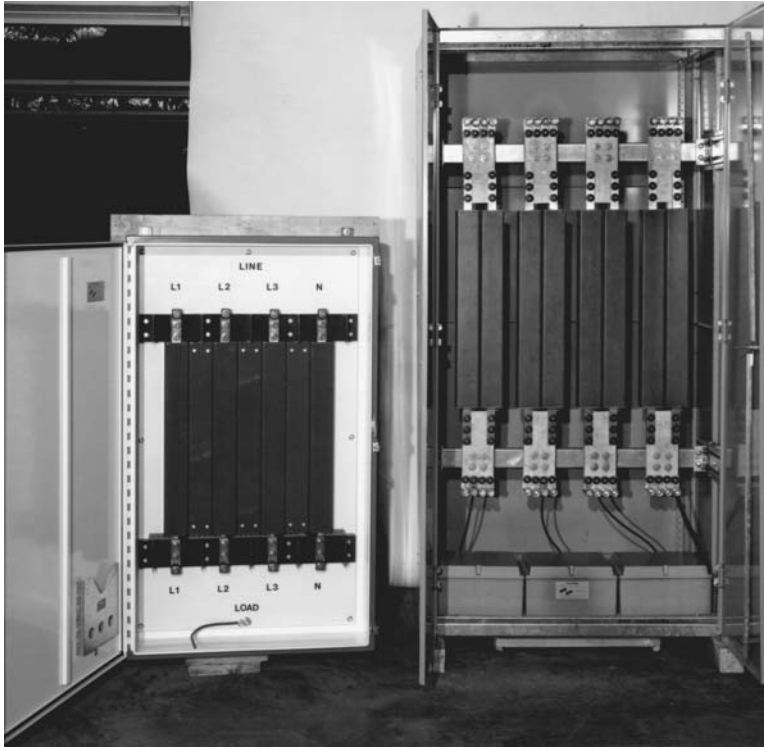
FIGURE 10.172 Interior view of a high-capacity hybrid power conditioner. (Courtesy of Control Concepts.)
