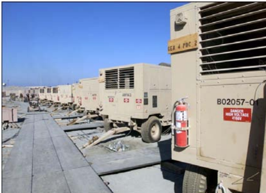
Figure 9.1. MEP-12 Power Plant.
