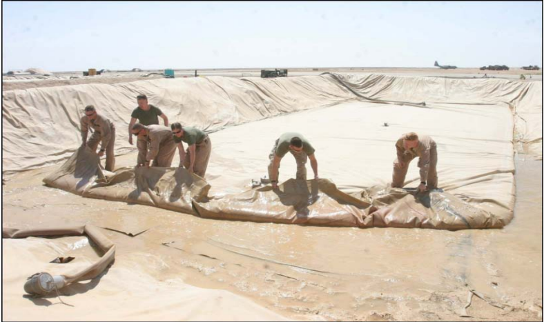
Figure 4.13. Fuel Dikes Control Spills and Forms Protective Barrier.
