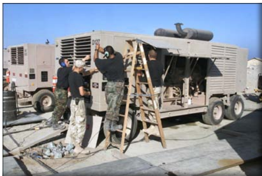
Figure 1.12. Preparing MEP-12 Generator at Forward Operating Location.
