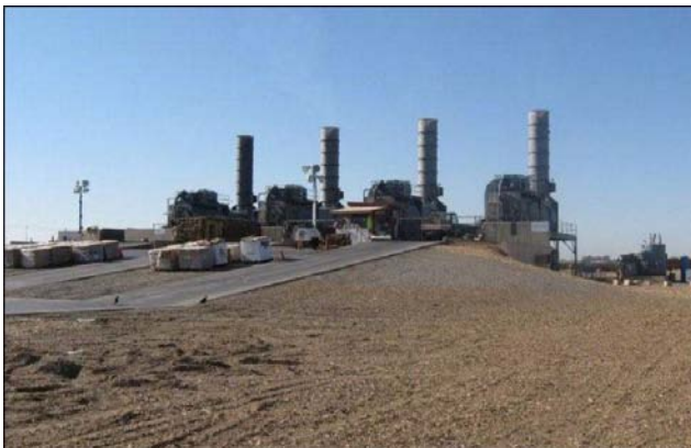
Figure 10.3. Incinerator Facility at Forward Operating Location.
