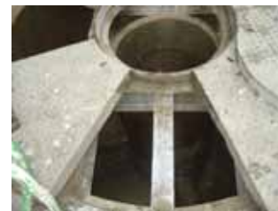
Figure 1. Outside view of grease trap
