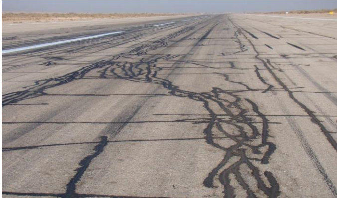
Figure 1. Overview of cracks in the Kerman Airport runway
