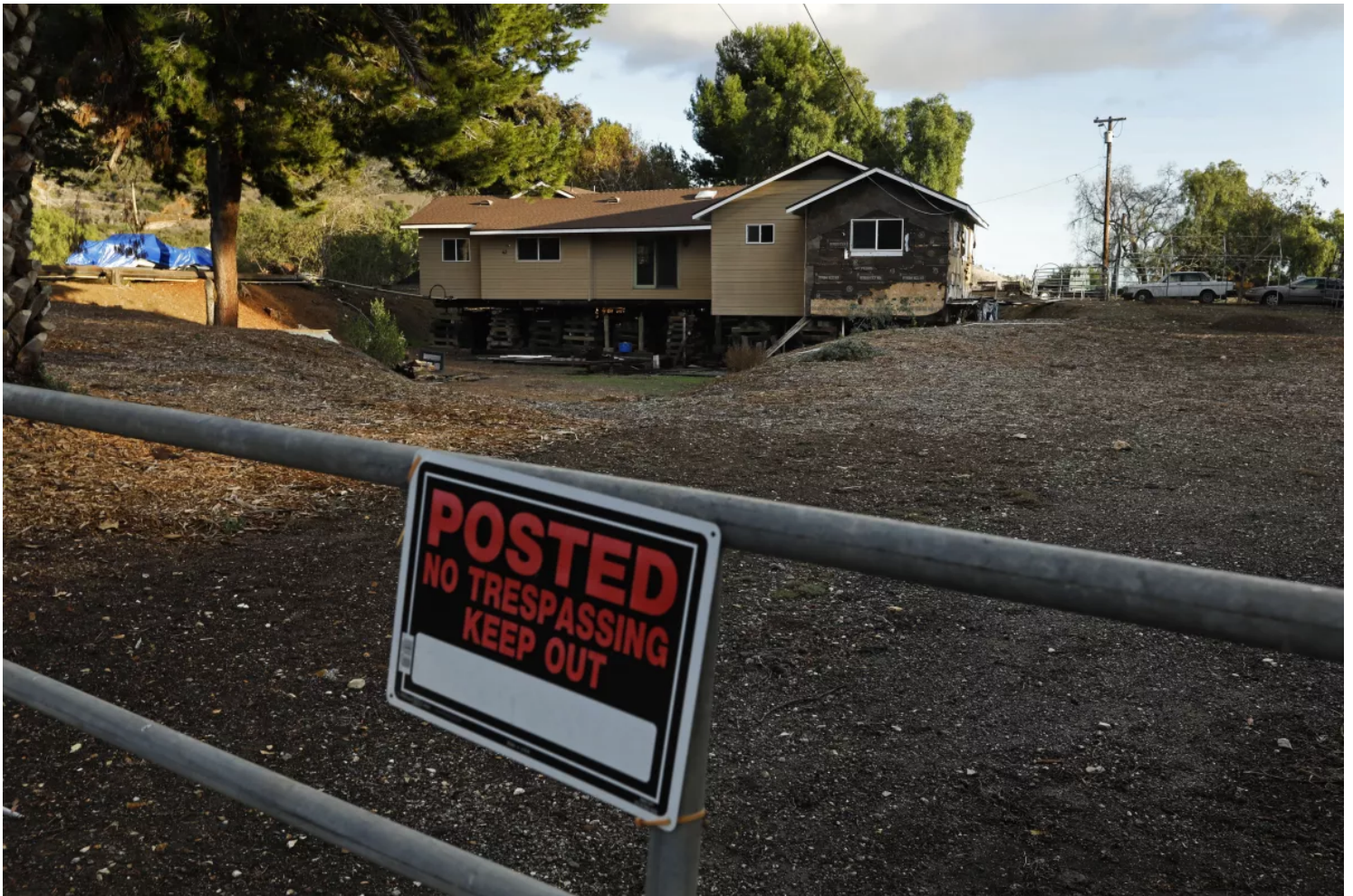
Some houses in Portuguese Bend are propped up on timber cribbing to keep the foundation steady with the shifting land. (Carolyn Cole / Los Angeles Times)
