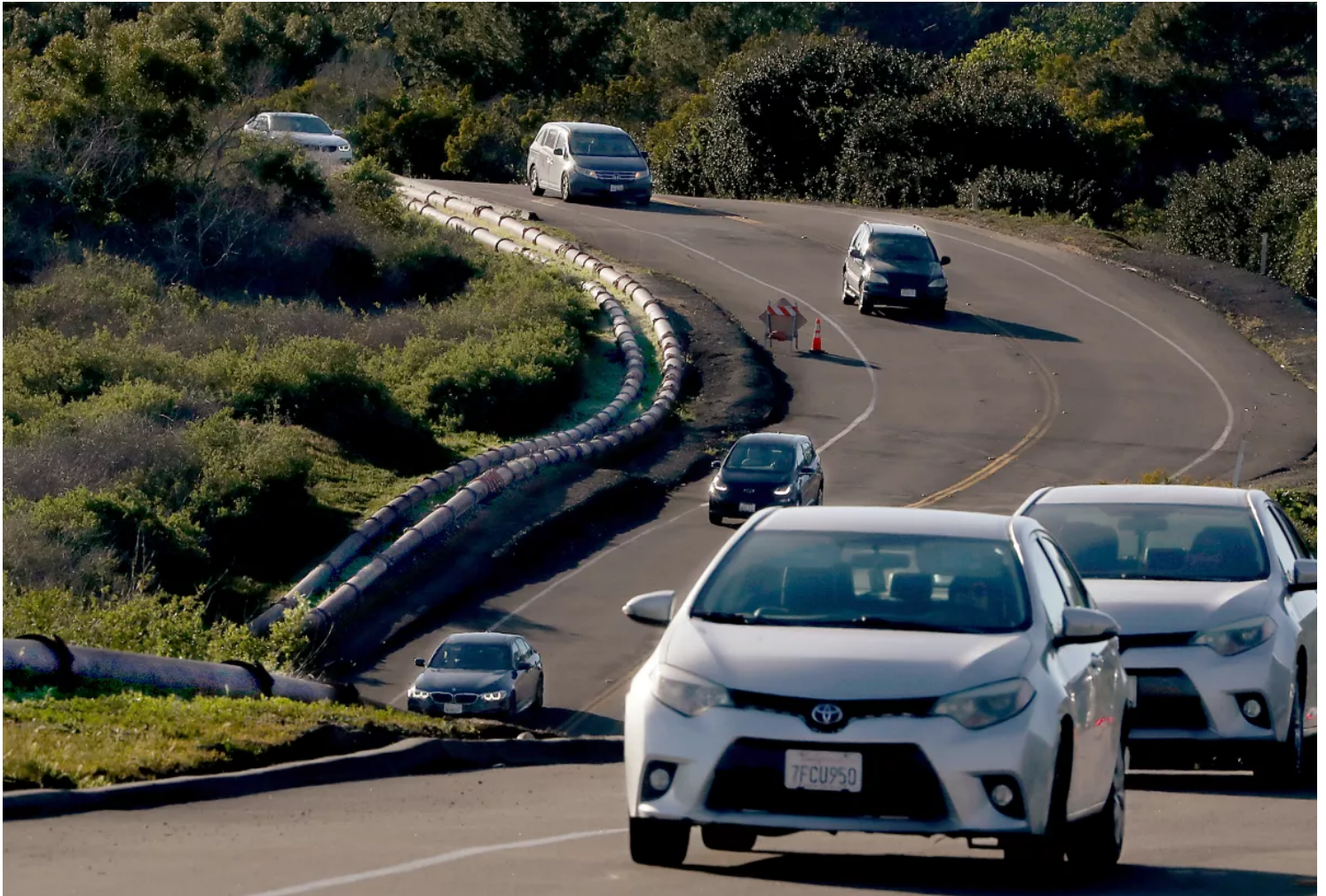
Sewage pipes run above ground along Palos Verdes Drive South at Portuguese Bend, where a stretch of roadway is uneven and erratic because of land movement on the coastline. (Luis Sinco / Los Angeles Times)
