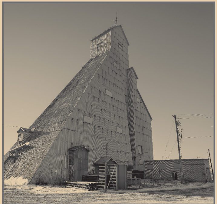
Photos of the McIntyre Headframe taken on December 02, 2020 by Lisa Romanowski. Thank you to Newmont Porcupine for permitting onsite access to the O'Gorman HS TGP3M Photography class.
