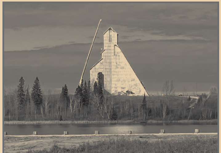
The crane is in place and work has begun on the McIntyre Headframe restoration. (Photo by Vera Romanowski.)
