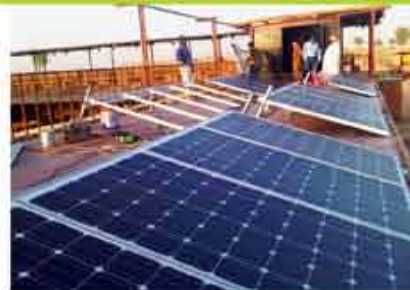
10KW Solar Power Project (100% Off-Grid System) Desert Safari Camp | Hatta South, Dubai
