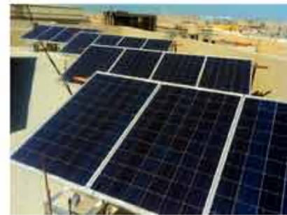
5KW Solar Power Project (100% Off-Grid System) Barsha South, Dubai
