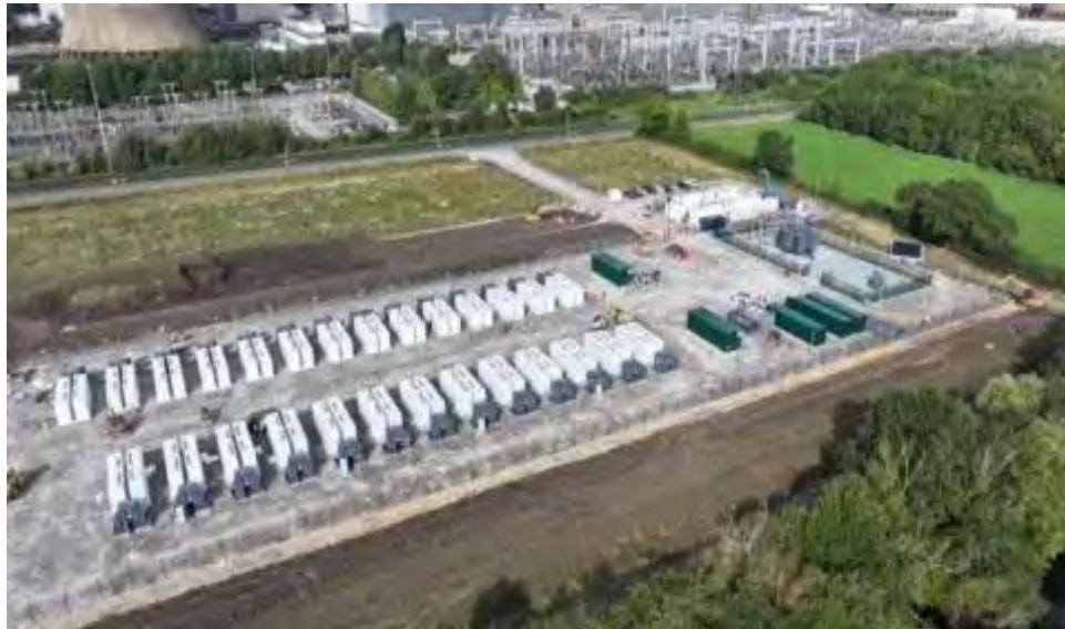
Lakeside Energy Park North Yorkshire, UK
