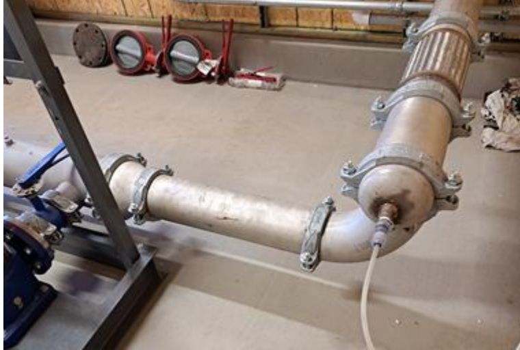
An example of grooved stainless-steel pipe with related fittings at a different water system.
