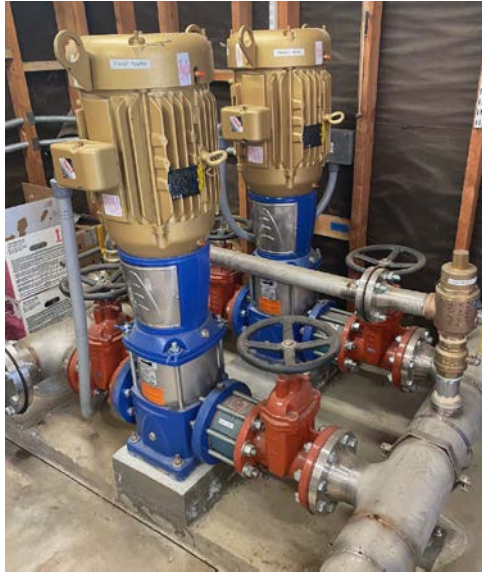
20 HP Variable Speed Booster Pumps
