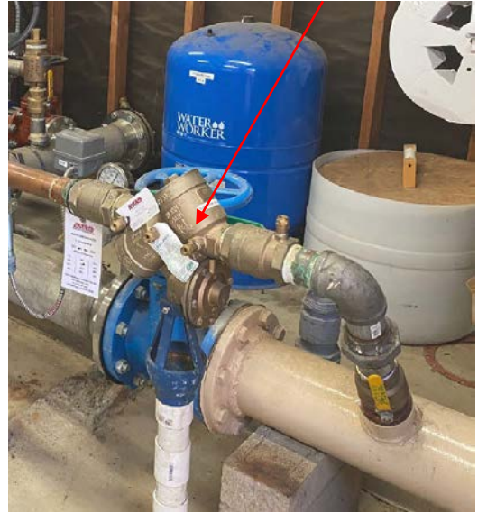
44 Gallon Pressure Tank w/ RP Backflow Device
