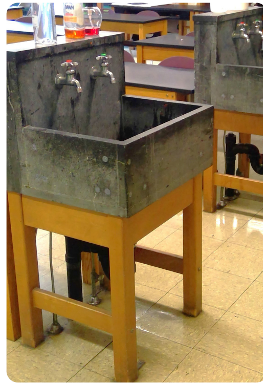
Plumbing fixtures not compliant per ADA (old!)
