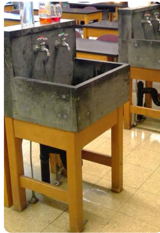
Plumbing fixtures not compliant per ADA (old!)
