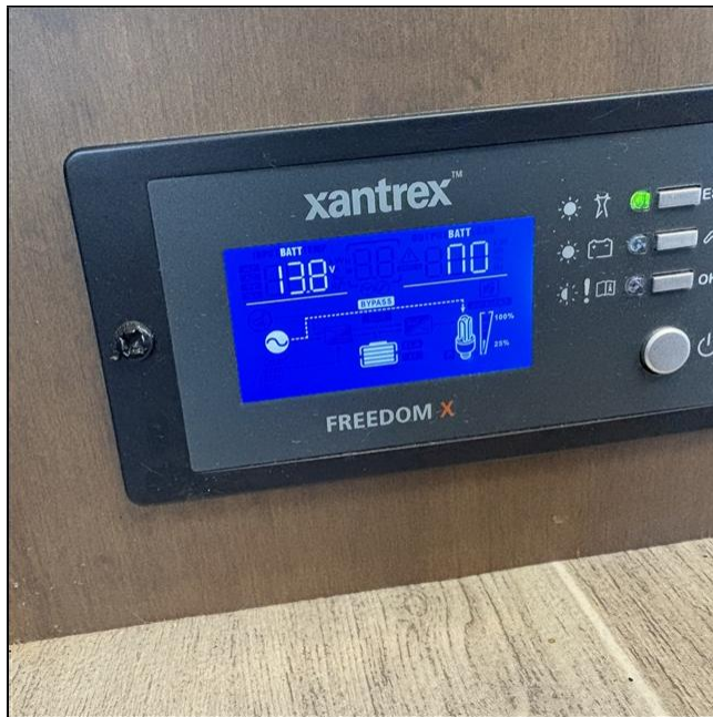
Plugged into shore power
