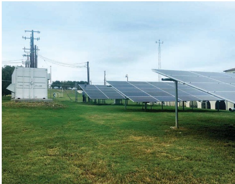
Demonstration microgrid at Joint Base San Antonio.
