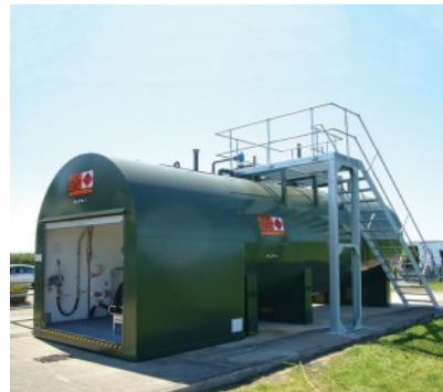
NEW BUNDED STORAGE TANKS UPTO 100,000 LTRS
