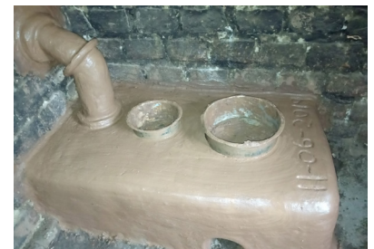
Clean cookstove being built. The stove's airtight cooking chambers and built-in chimney ensure that smoke is not released into the home.
