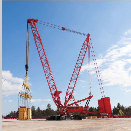
MANITOWOC MCL650 WITH VPC-MAX 772- Tons Capacity Triple Heavy Duty Spreader Bar with 100' Spread 1,354- Ton Lift of Building Steel Foundation in 2 Sections (677-Ton Lift Per Section) 166-Ton Steel Plate in 2 Section (83-Ton Lift Per Section)
