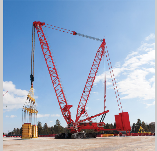
MANITOWOC MCL650 WITH VPC-MAX 772- Tons Capacity Triple Heavy Duty Spreader Bar with 100' Spread 1,802- Ton Lift of Building Steel Foundation in 3 Section (600-Ton Lift Per Section 235-Ton Steel Plate in 3 Sections (78.3 Tons Lift Per Section)
