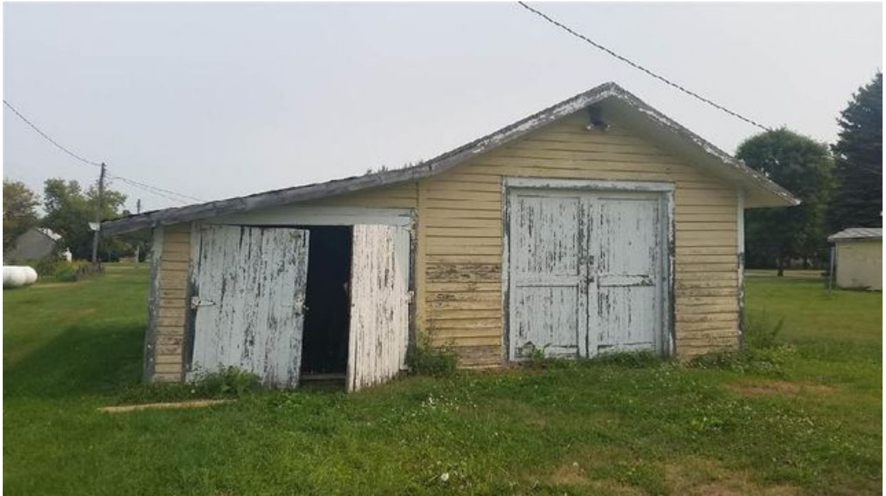
GARAGE NEEDS SOME WORK TO BE TURNED INTO GRANT COUNTY ND NEWS DOT COM OFFICE SPACE
