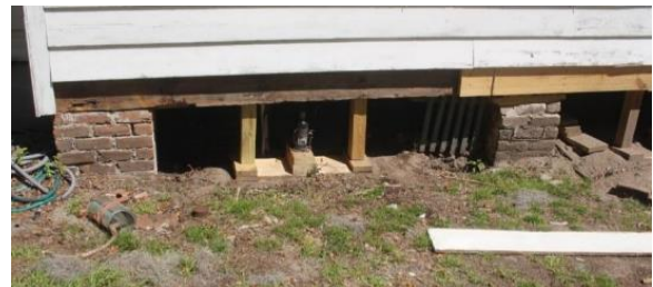
Detail of the work to level the building. Note the screw jack.
