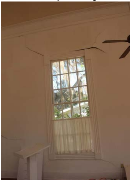
The damage is evident in this photo.
