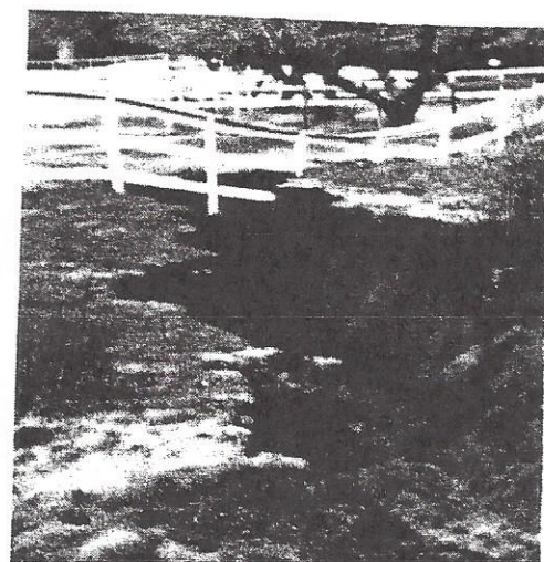
EROSION CUTS LAND IN HALF
