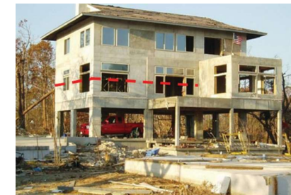
The water line was at 28 ft. as indicated by the red line in this photo.
