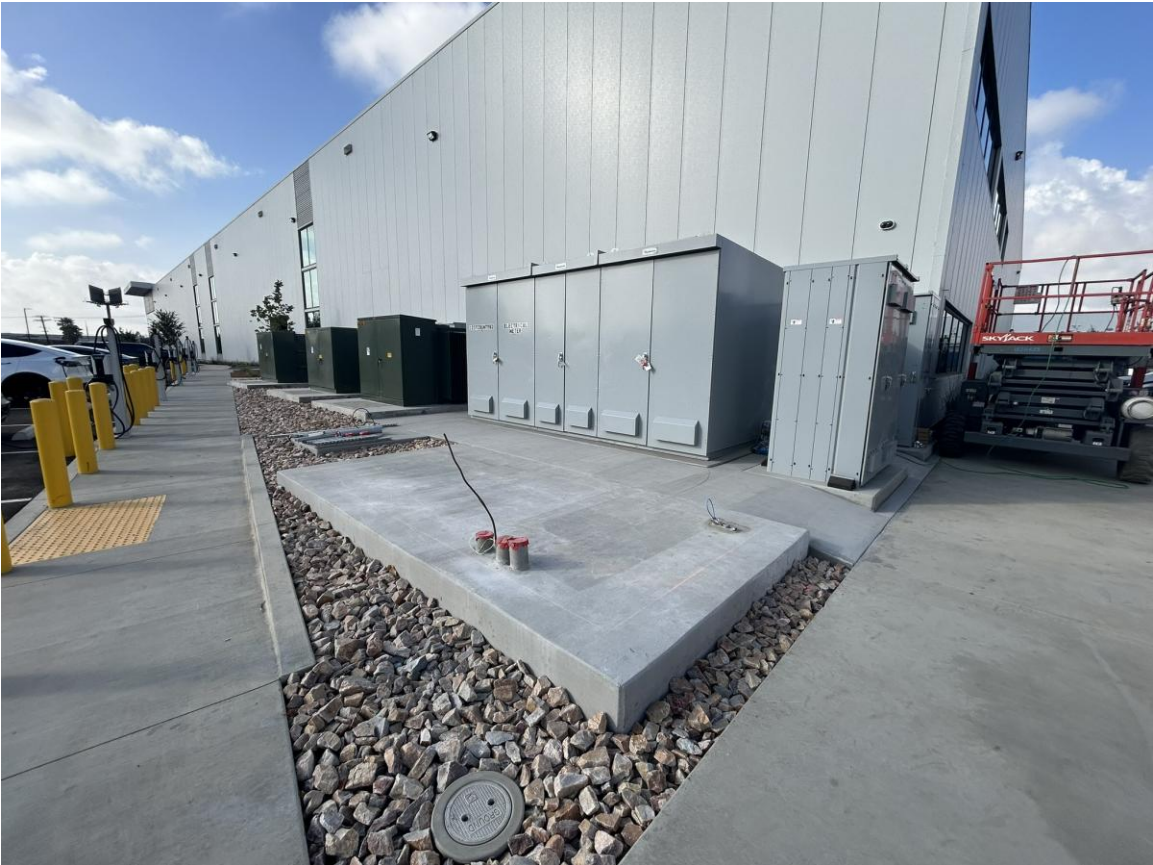
Electrical utilities shown without BESS; storage installation remains pending.
