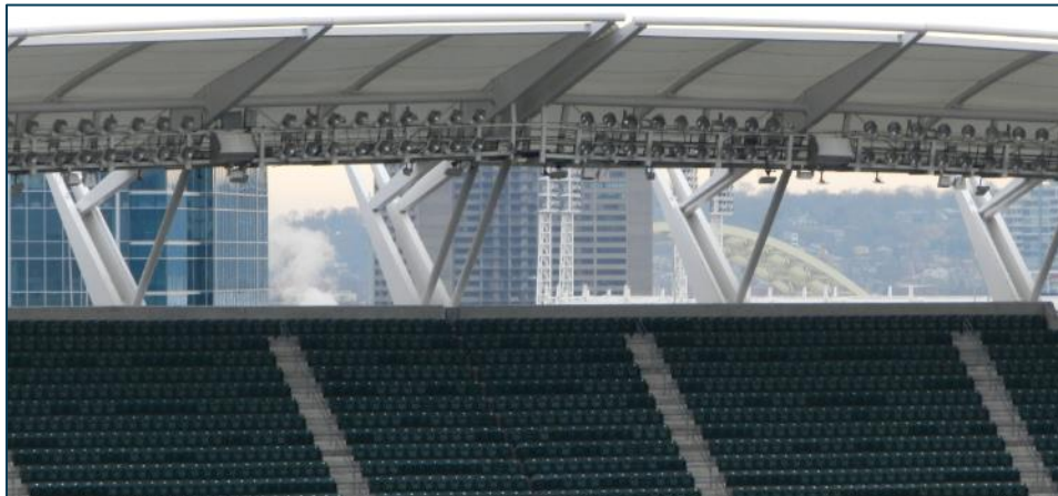
ORIGINAL FIELD LIGHTING AT PAYCOR STADIUM (TOP ROW AND BOTTOM ROW)
