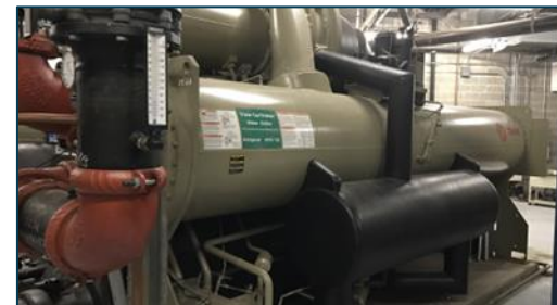
CHILLER AT THE JUSTICE CENTER
