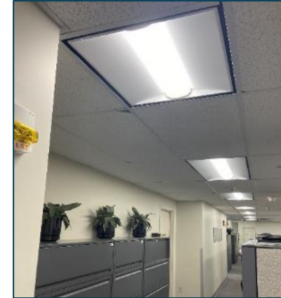
LED FIXTURES AT ADMINISTRATION BUILDING
