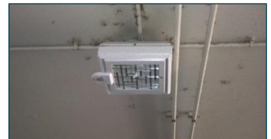
NEW PARKING GARAGE LED LIGHT FIXTURE
