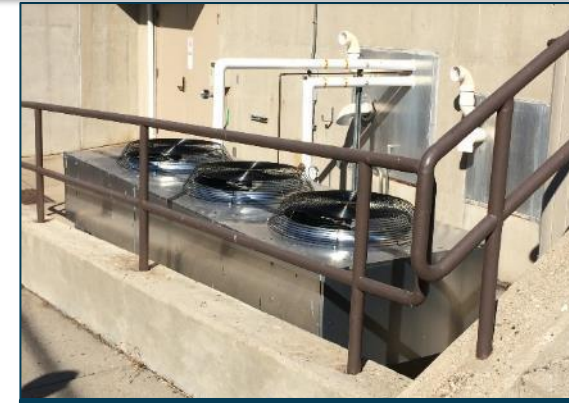
FLUID COOLER AT 911 COMMUNICATIONS
