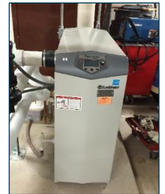
CONDENSING WATER HEATER AT JUVENILE DETENTION CENTER
