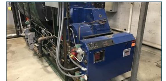
BOILER BURNER AT THE COURTHOUSE
