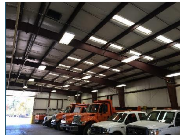
HIGHBAY LIGHTING AT PUBLIC WORKS GARAGE
