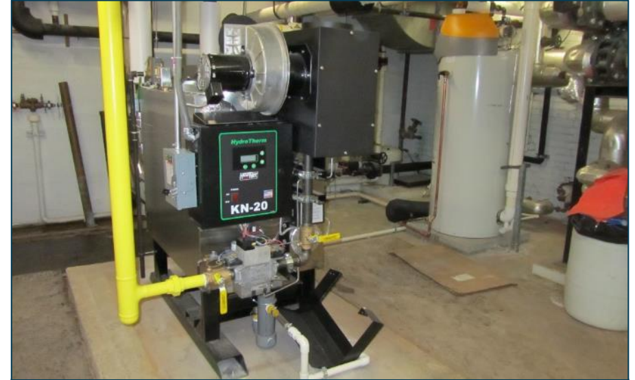
NEW CONDENSING BOILER INSTALLED AT 203 E. 9 TH ST
