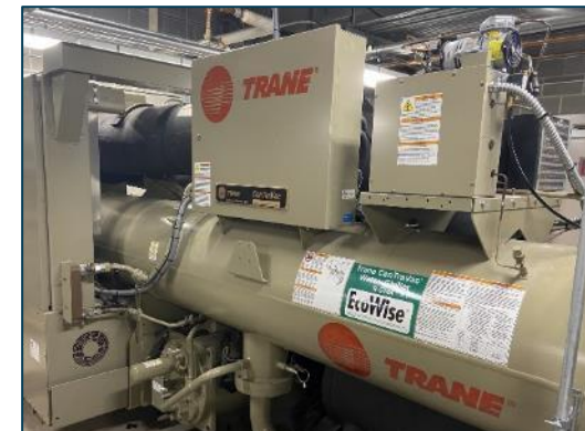
CHILLER AT JUVENILE DETENTION CENTER
