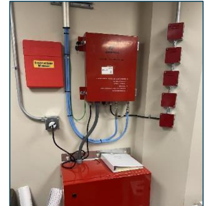
FIRE ALARM SYSTEM AT PORTUNE CENTER
