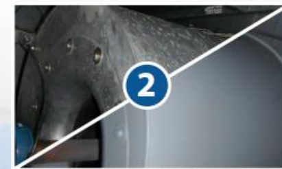
Blower Unit After PURE-Coat
