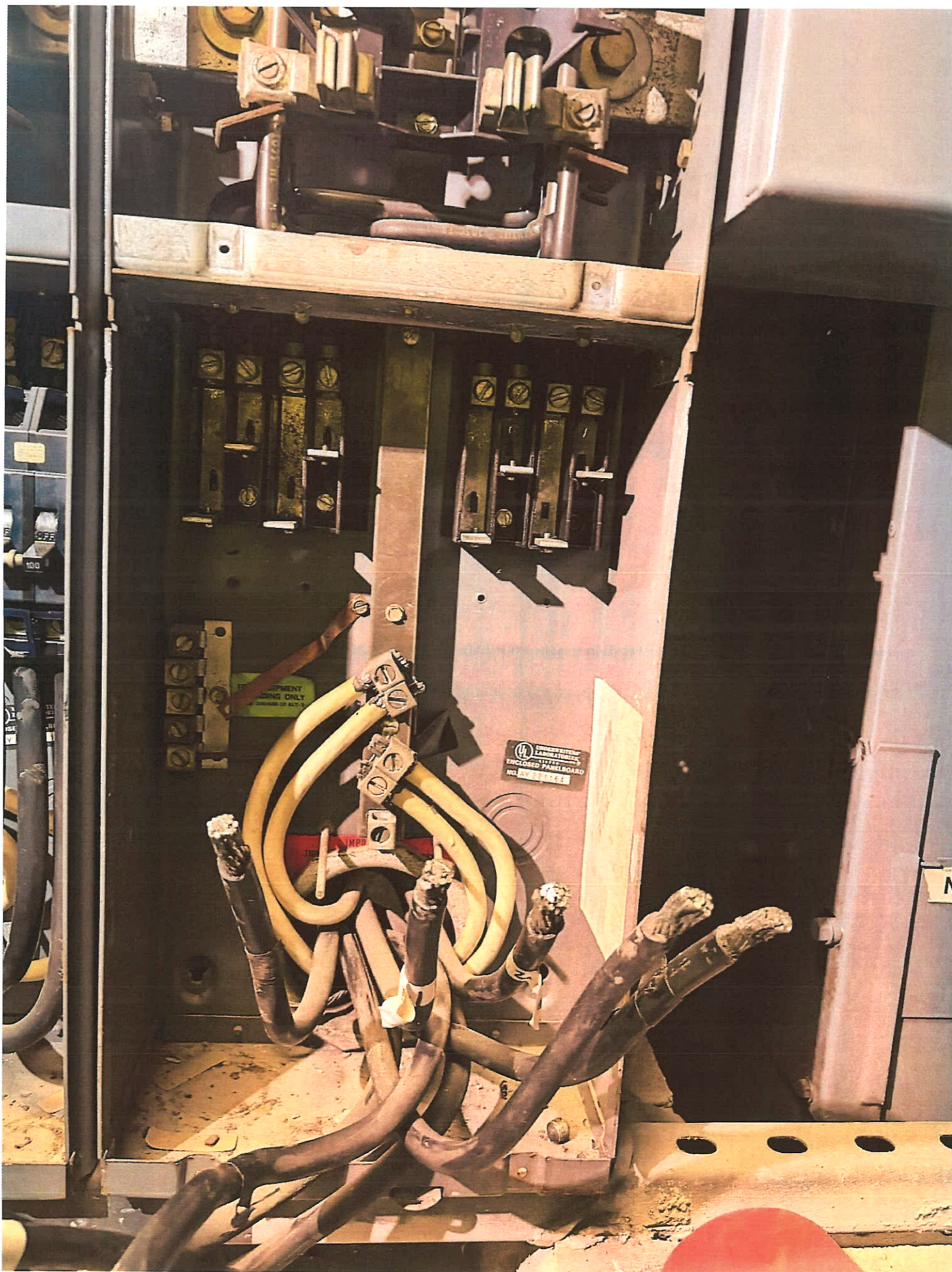
METER CENTER GUTTED
