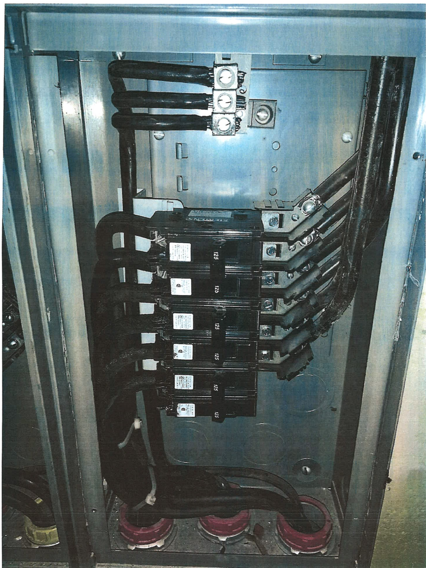
RETRO FIT TO SIEMENS
