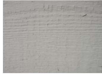
Paint surface already cracking.
