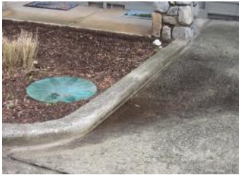
Section of concrete driveway maybe draining slowly.
