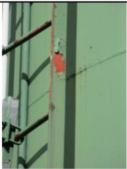
Water tank finishes must be regularly and properly maintained.
