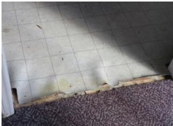
Flooring in poor condition.
