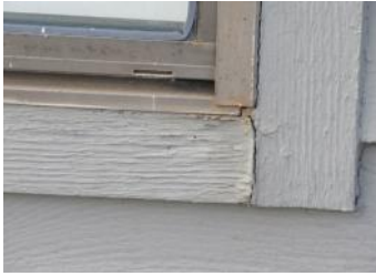
Building surface in poor condition. Sealant no longer functioning.
