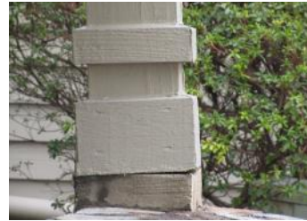
Deck post leaning.
