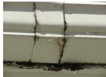
Leaking gutter and likely rot of fascia board.
