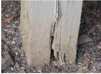
Rotting deck post.
