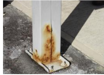
Mailbox post exhibiting severe rust.
