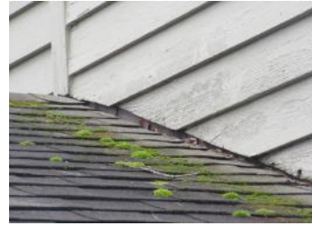
Moss should not be growing on shingles.
