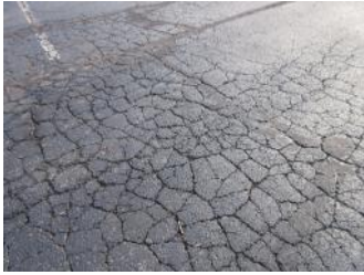
Parking lot exhibiting alligator cracking.
