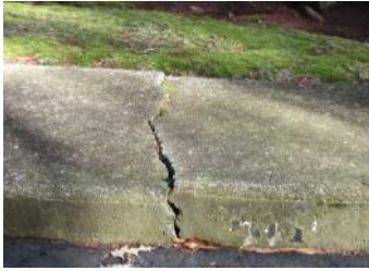
Minor concrete damage found.
