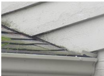
Siding should not be in contact with shingles.
