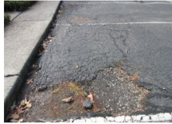
Parking in poor condition.
