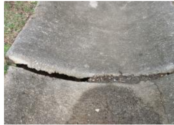
Void under storm curb has formed.
