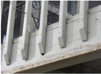
Paint has peeled.
