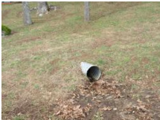
Galvanized metal pipe will eventually rust.
