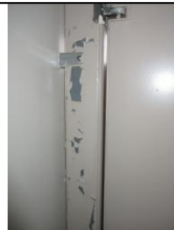
Toilet partition finish has failed.
