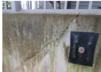
Retaining wall tiebacks. Couldn't determine if cracking formed before or after installation.
