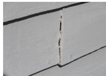
Movement in siding and cracked caulk.
