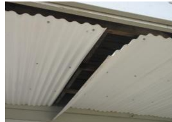
We advocate against covering deck undersides.
