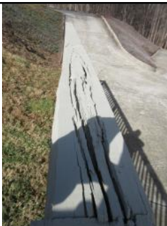
Some repairs, especially horizontal members should be performed periodically.
