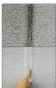
Top photo: The weather sealants used in the EIFS cladding at Michigan's Kelsey-Hayes World Headquarters building has dried, cracked and failed. Bottom photo: DOW CORNING 123 Silicone Seal was applied, opening the old weatherseal, followed by a coat of ALLGUARD® Elastomeric Waterproof Coating from Dow Corning.
