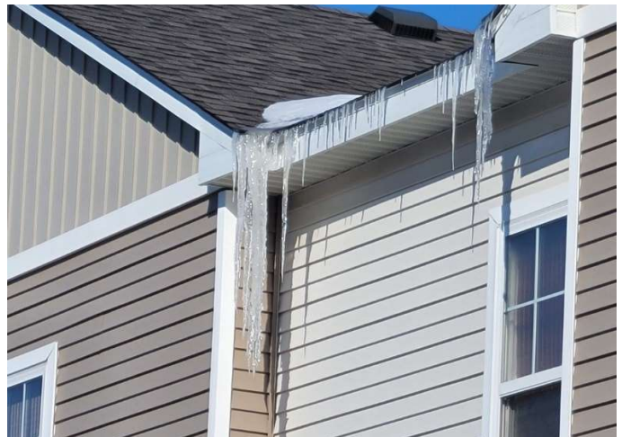
Ice damming at eave
