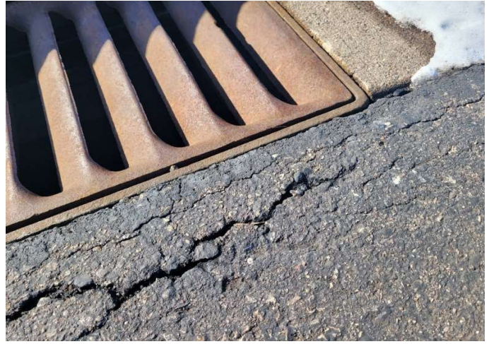
Settlement and cracks near catch basin
