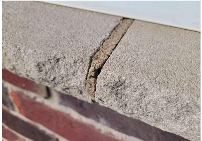
Cracked mortar joint between sill sections
