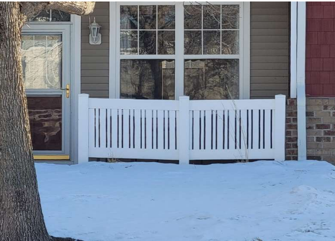
Heaved fence post; Unlevel fence
