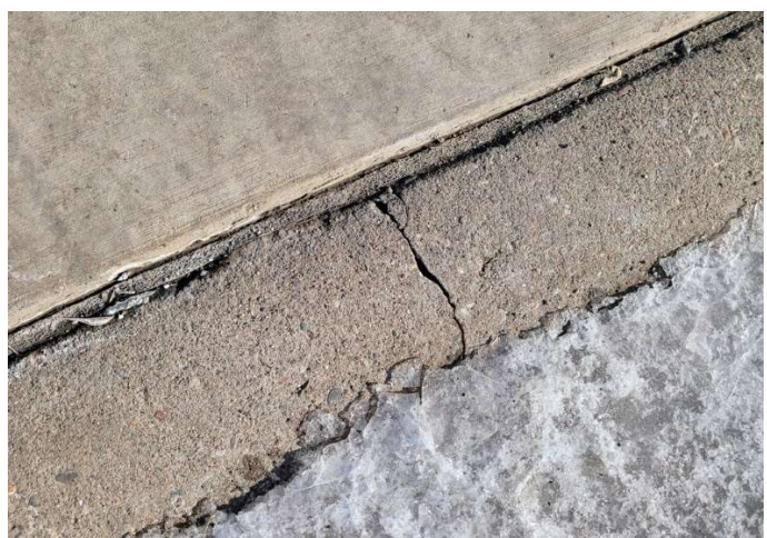
Crack at concrete gutter
