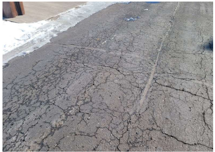
Severe fatigue cracking
