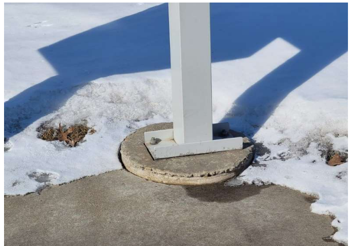
Pedestal base at mailbox station
