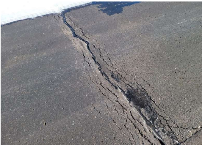
Crack at pavement
