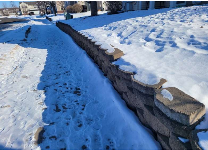
Overview of retaining wall with slight lean
