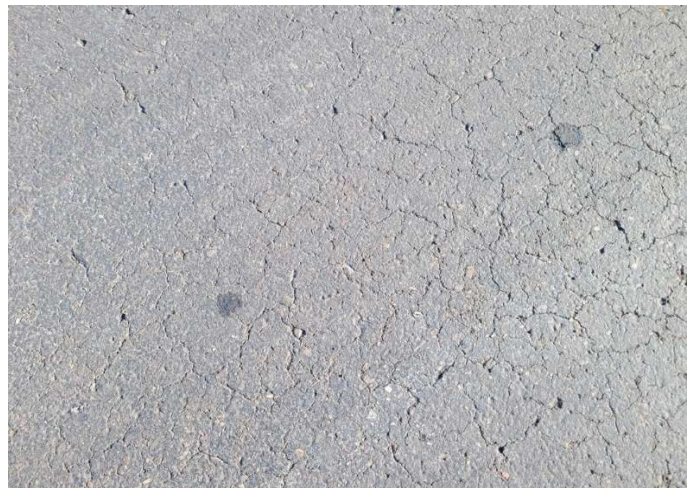
Surface condition at asphalt pavement
