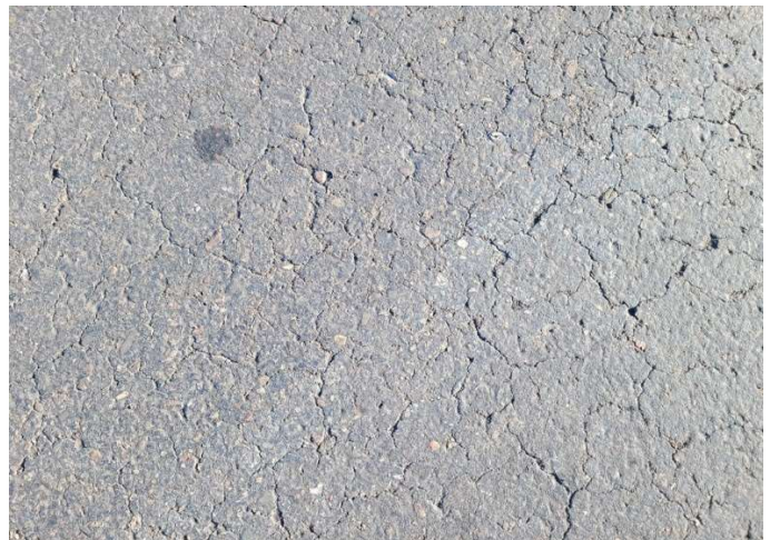
Surface condition at asphalt pavement
