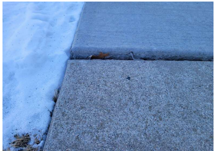
Isolated condition of trip hazard at unlevel walk
