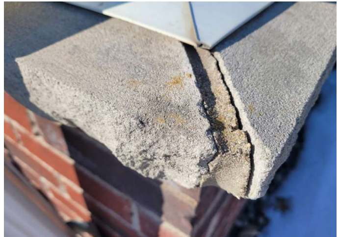
Cracked mortar joint at exterior sill corner
