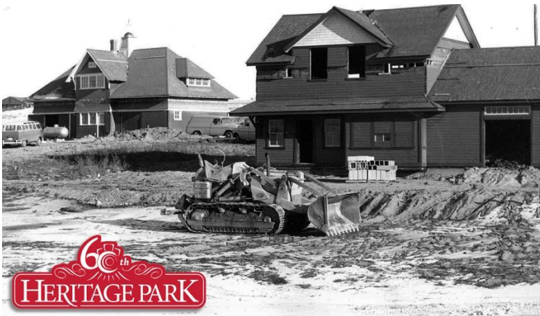
Construction of Midnapore Station and Hull Carriage House. Heritage Park Historical Village, Courtesy of Pat Turner
