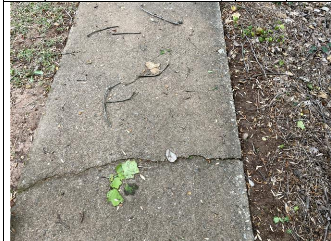
Cracked sidewalk example
