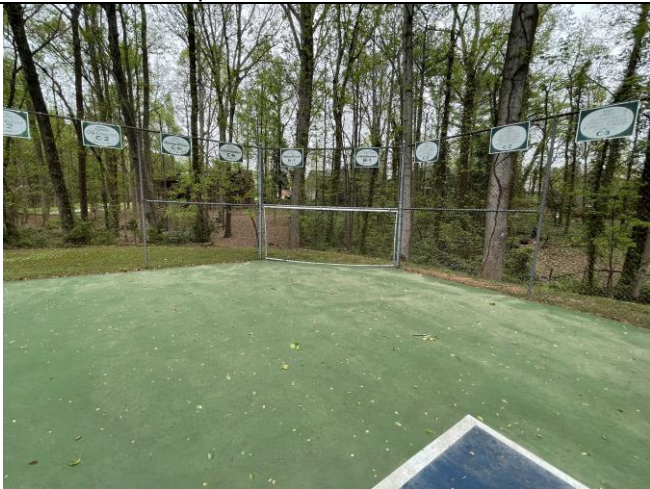
A section of the fence has been replaced
