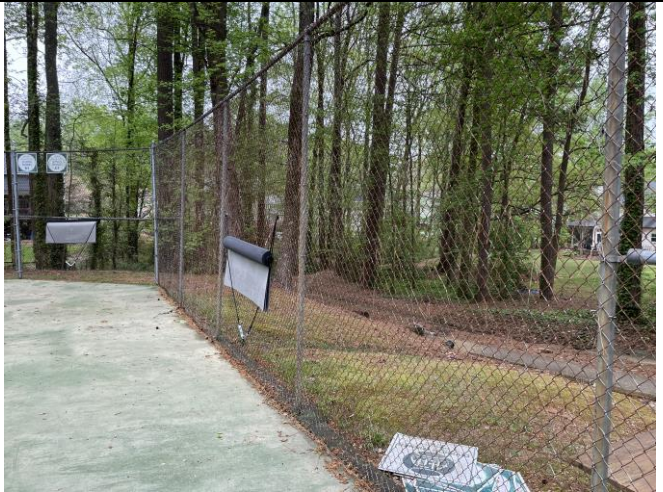
Example of the corroding fence
