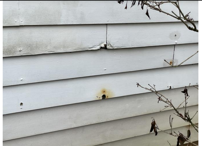
Siding swelling at edge and nail holes
