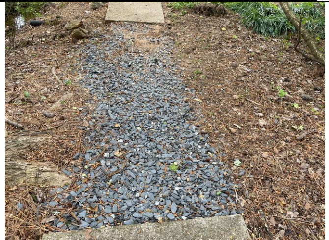
Section of sidewalk missing
