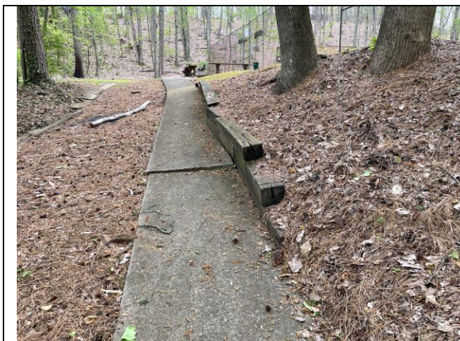
Wall bowing and leaning
