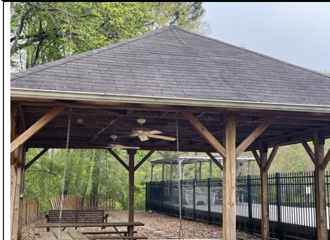
Pavilion with missing shingles
