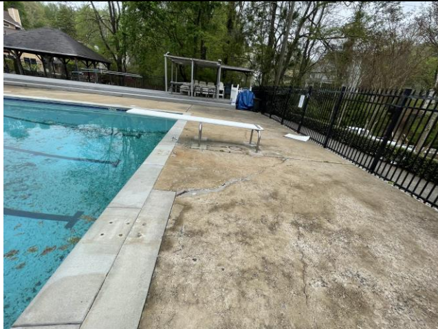
Pool decking with recent pool edge repairs
