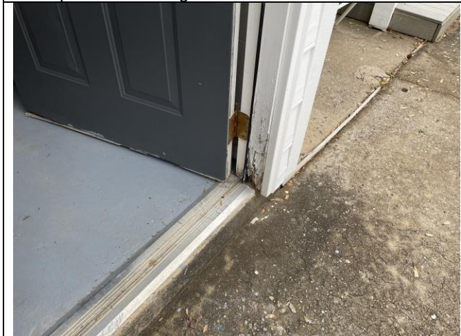
Example of damage at door trim
