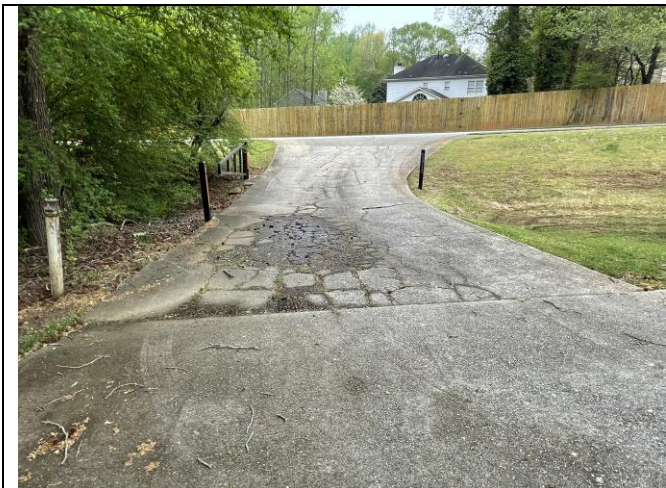
Damaged driveway to parking lot
