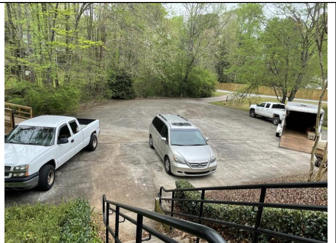
Cracks visible in the parking lot
