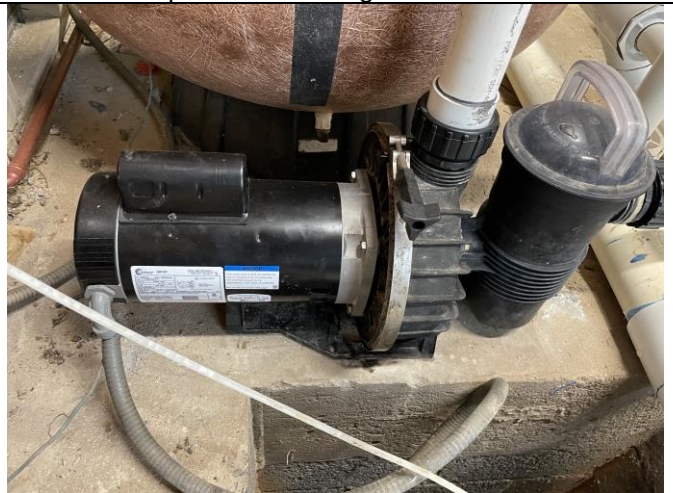
One of two 3 HP pumps
