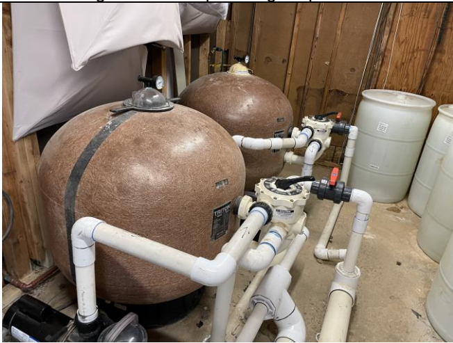
Two filters with two pumps
