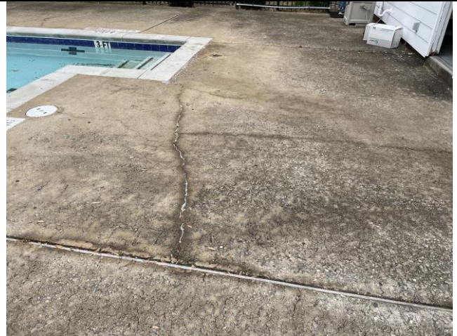
Cracks in the pool side decking
