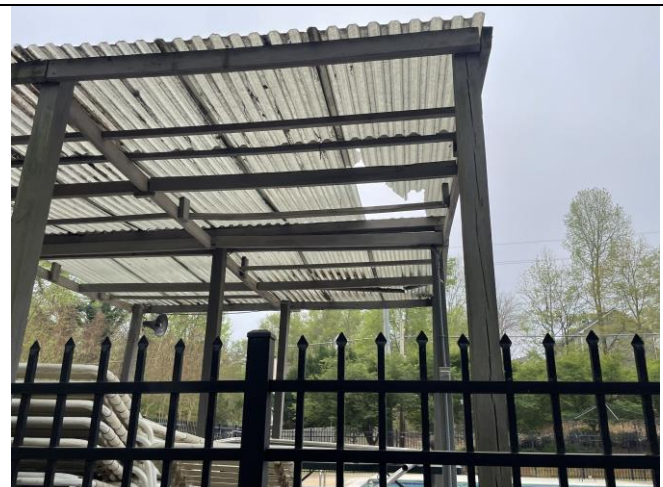
Damage to the Gazebo roof
