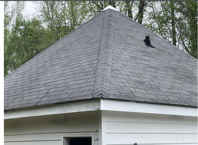
Poolhouse roofing. Note: no gutters
