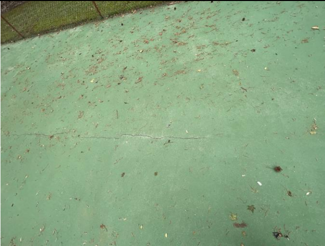
Small crack at a perimeter
