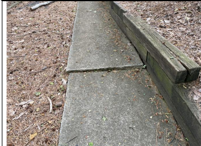
Example of shifted/settled sidewalk (trip hazard)
