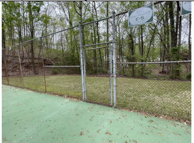
Corroding of galvanized post and fence evident
