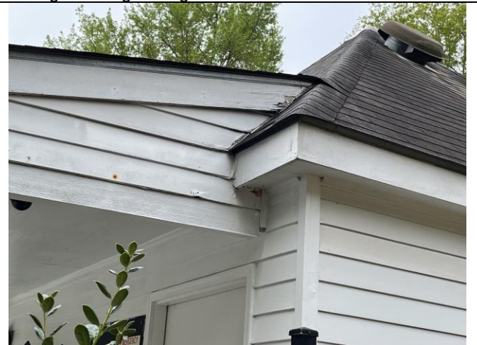
Example of siding and trim damage
