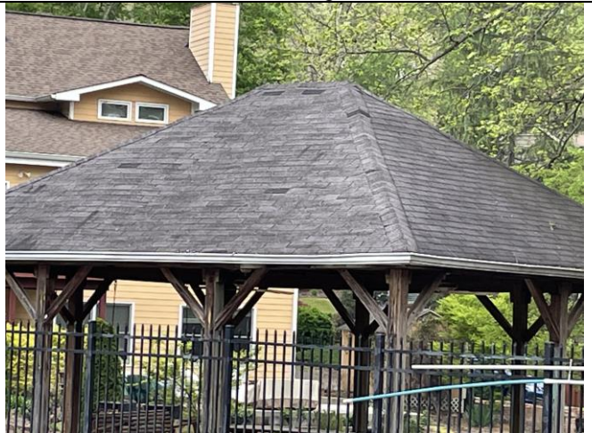
Pavilion roof with several damaged shingles
