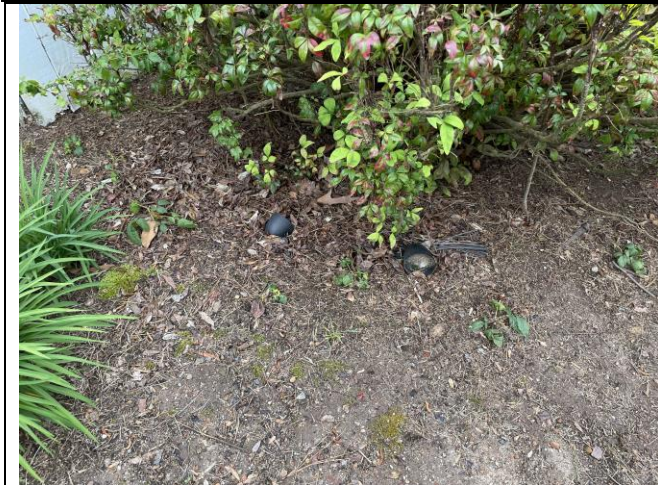
Landscaping lighting damaged
