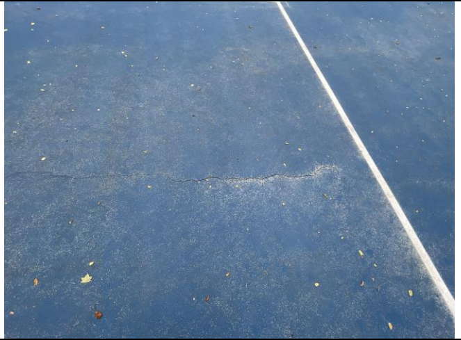
Small crack in the court area
