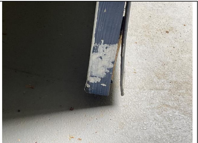
Outside panel coming off at ladies' bathroom door
