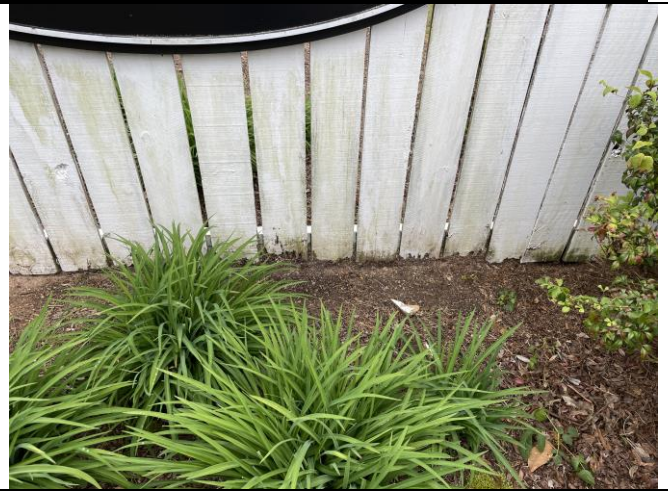
Signs of deterioration at the base of the pickets
