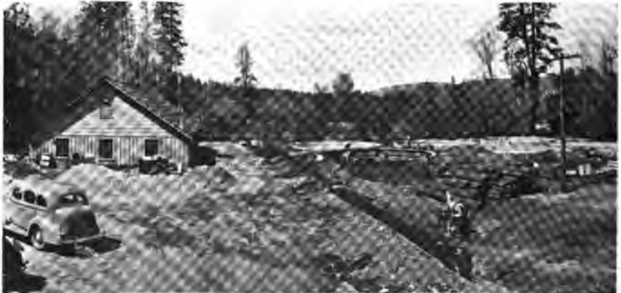
Panorama view of new Spokane hatchery construction. (Left) Hatchery building. Seventeen standard 40-foot concrete rearing pools are now in operation here.
