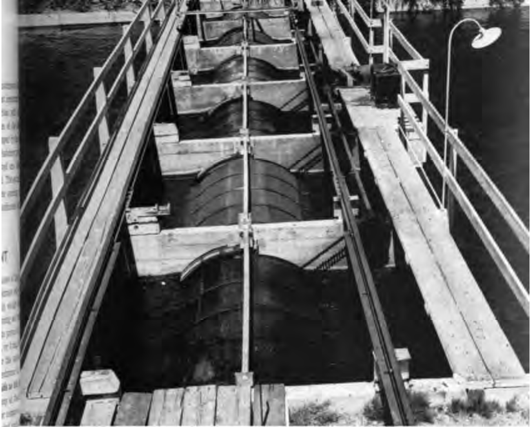
A typical fish screen constructed to prevent fish from being lost in an irrigation project.
