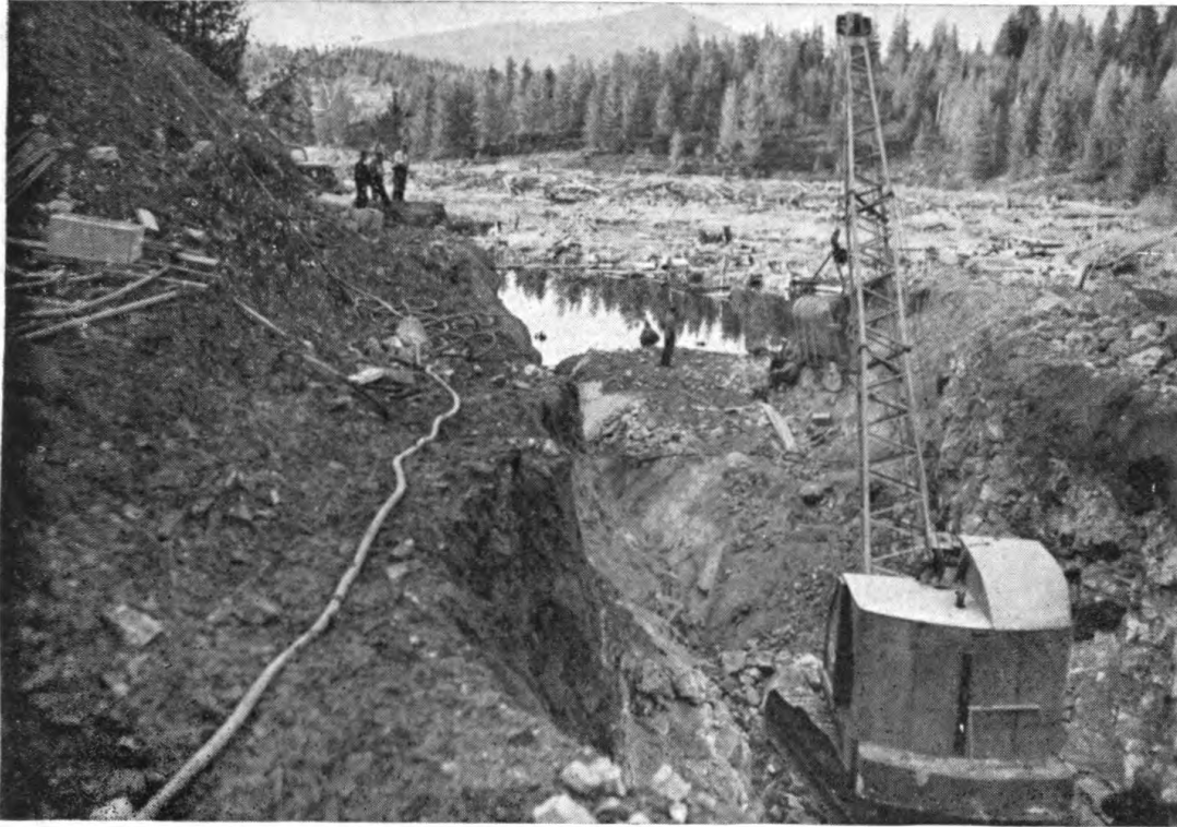
Power shovel digs spillway for Elk creek dam. Game department is restoring a mile-long reservoir, which was once a heavy producer of eastern brook trout. This large construction project was let on bid to a contracting firm.
