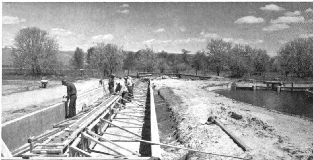
Workmen remove forms from new concrete rearing ponds at the Eagle Hatchery. Two new wells were also placed in operation at this hatchery during the biennium.
