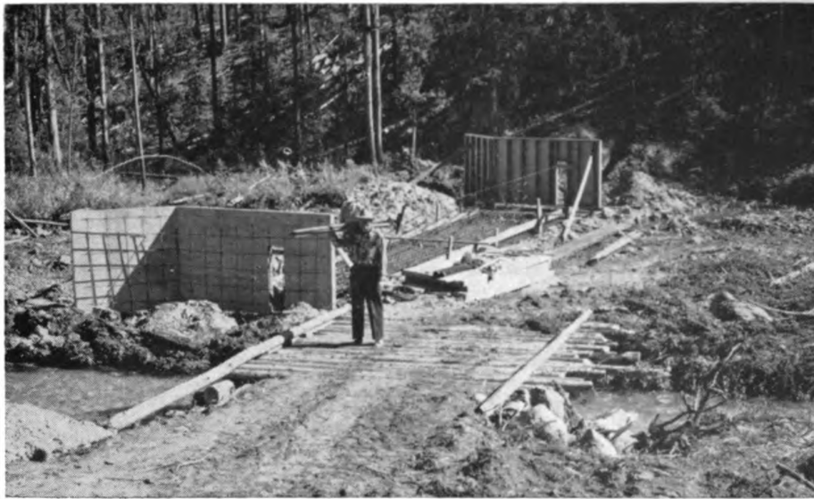
A migration-block dam was constructed at the outlet of Stanley Lake to prevent fish from moving upstream into the lake after it was stocked with game fish.
