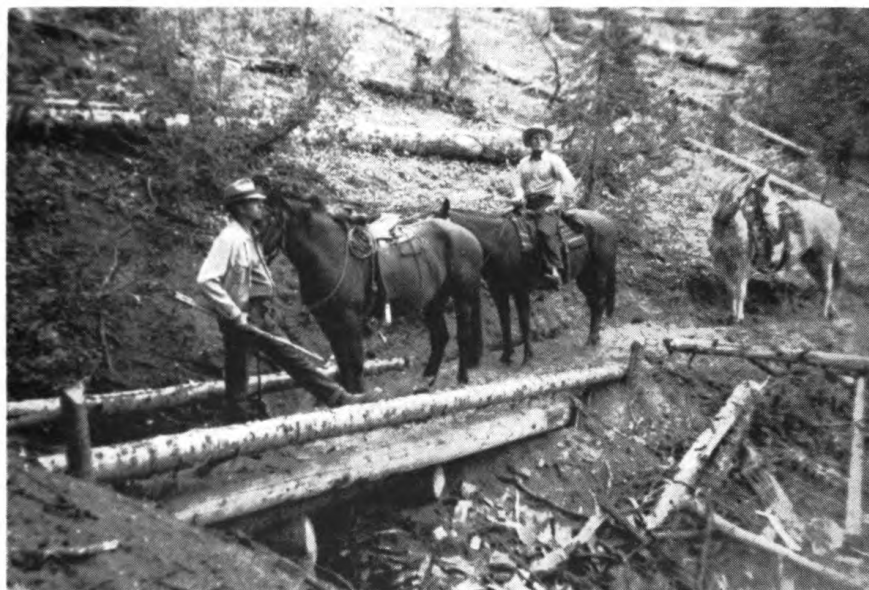
A section of new fisherman access trail that was constructed to mountain lakes in the Sawtooth Wilderness Area during the biennium.
