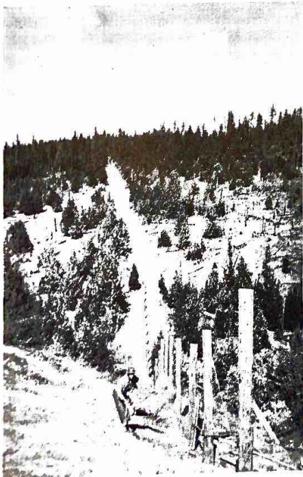
Part of a five-mile fence built by the game department's construction crews. The barrier encloses white-tail deer study area, was eight feet high and required 2,100 posts. (F&G Photo)
