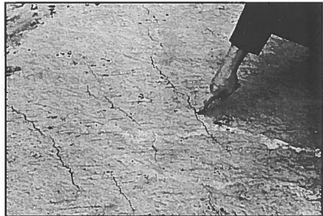
Plastic Shrinkage Cracks
