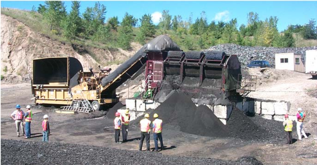
Picture 14 - Shingle Grinder Followed by Trommel Screen
