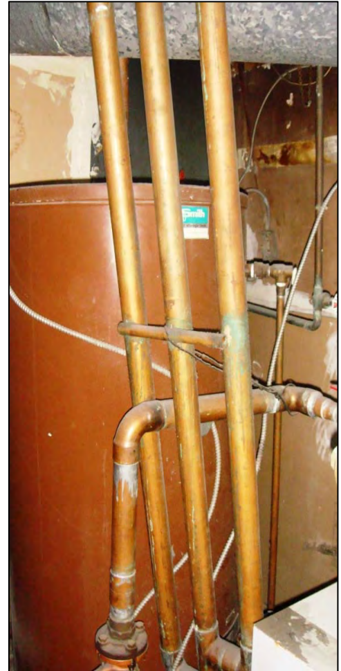
Photo 7: View of the furnace and hot water tank located in the laundry facility
