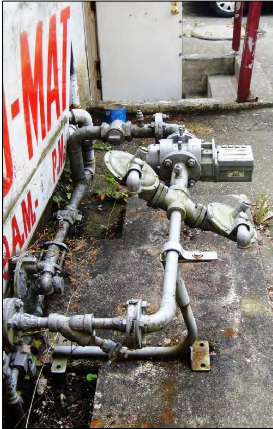
Photo 4: View of the gas meter in the rear of the laundry facility at 4227-31 E. Hastings. Looking W.
