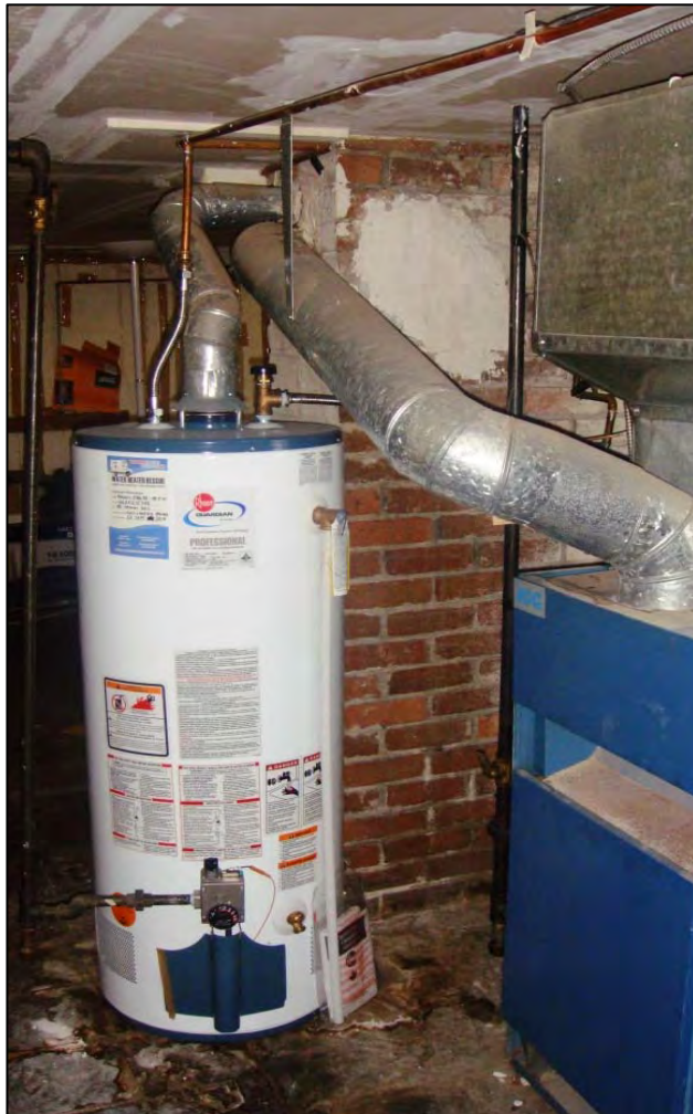
Photo 8: View of the residential natural gas furnace and hot water tank located in the basement. Looking NE.
