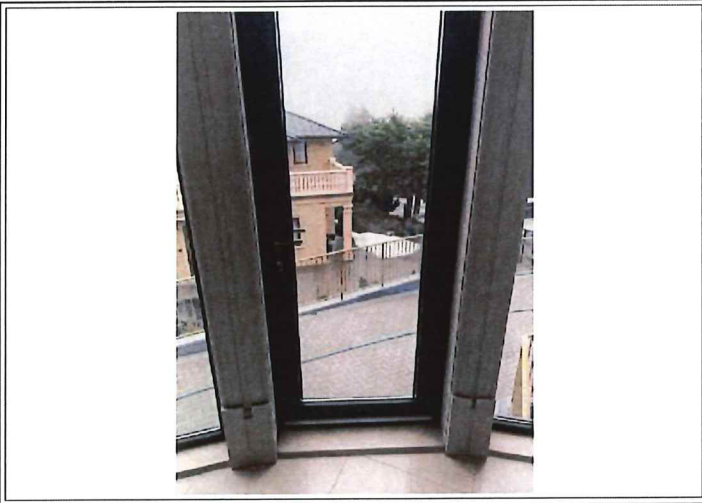
FRENCH DOOR IN OFFICE: NOT SECURE AND NO DECK BUILT OFF OF IT
