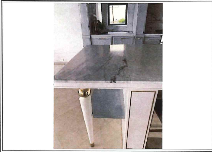
SHALLOW STONE SLABS ON ISLAND POORLY MATCHED/POORLY FINISHED
