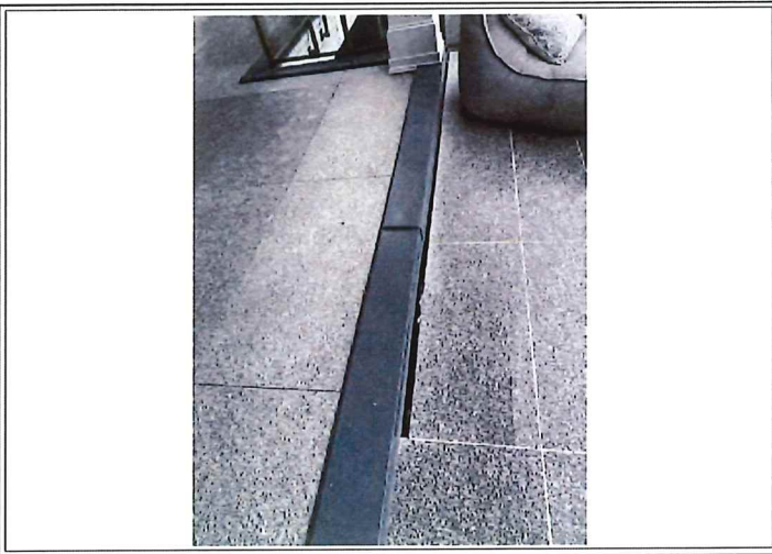
FLASHING USED AS TRANSITION STRIP AND GAP UNCOVERED
