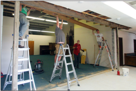
Workers install a beam as part of the renovation of the lobby/mercantile.
