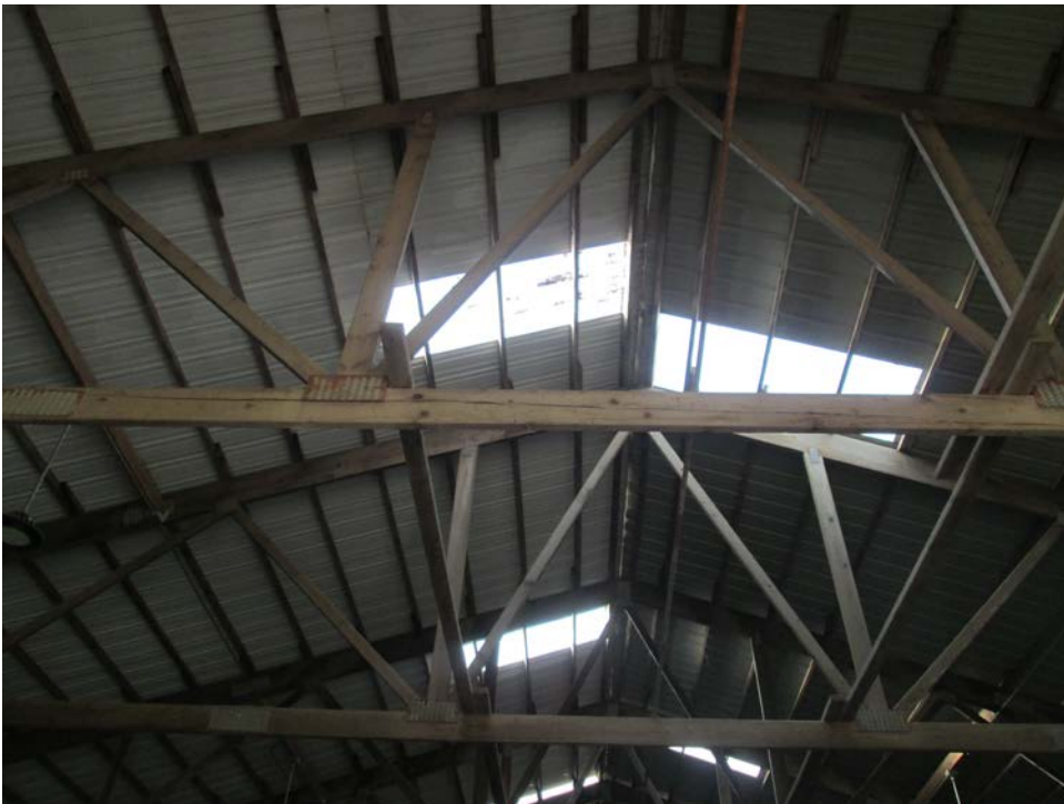
Photo 2 Cracked Truss Bottom Chord at West Barn
