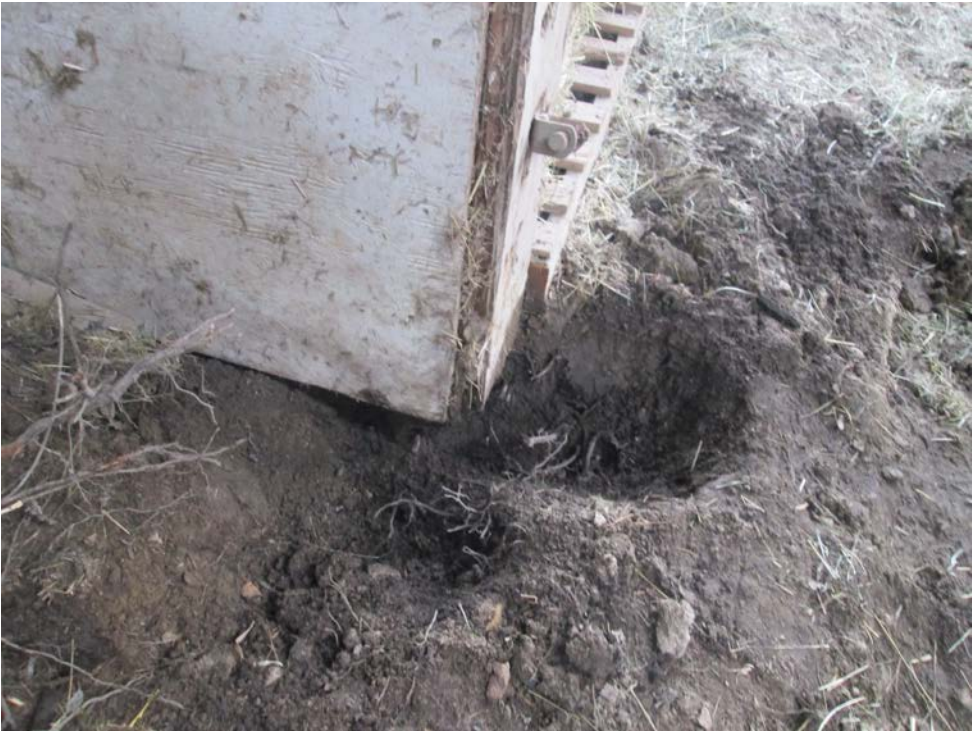
Photo 6 Rotting Interior Column Base at East Barn Building
