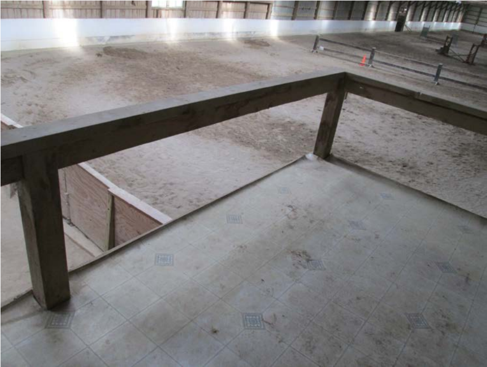
Photo 5 Non-Code Compliant Railing at Judging Platform
