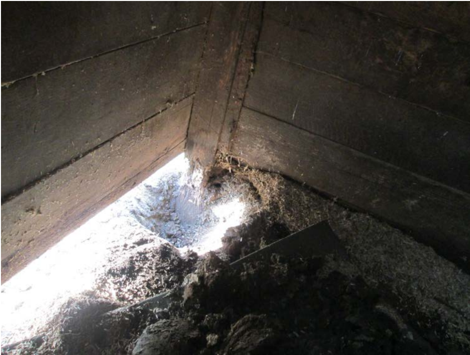
Photo 9 Deteriorated/ Missing Column Base at East Barn Building
