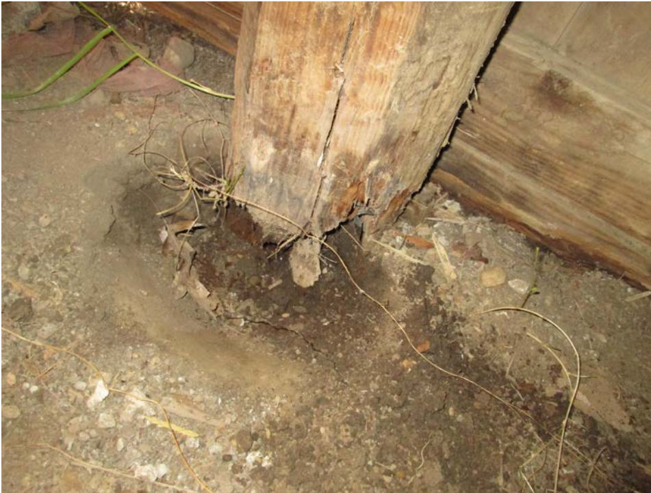
Photo 11 Rotted Column Base on East Wall of West Barn Building
