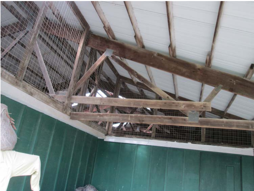
Photo 4 Cut Truss Bottom Chord at West Barn Cross Gable Roof
