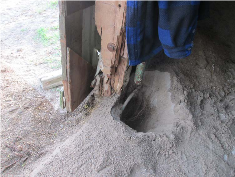
Photo 7 Deteriorated Jamb Column at North Wall of West Barn Building
