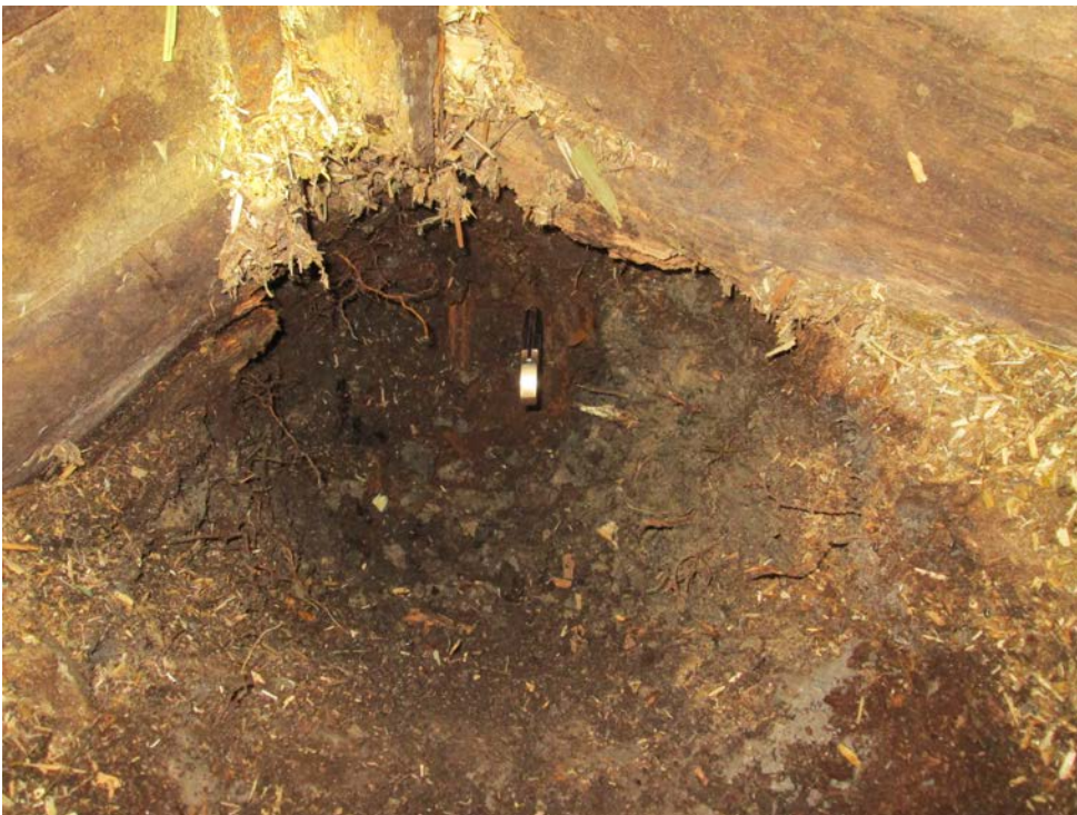
Photo 10 Rotted Column Base on East Wall of West Barn Building
