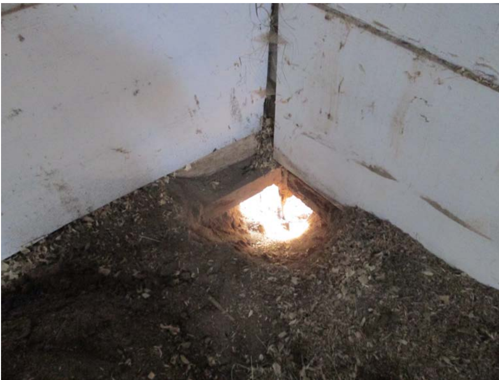
Photo 8 Deteriorated/Missing Column Base at East Barn Building
