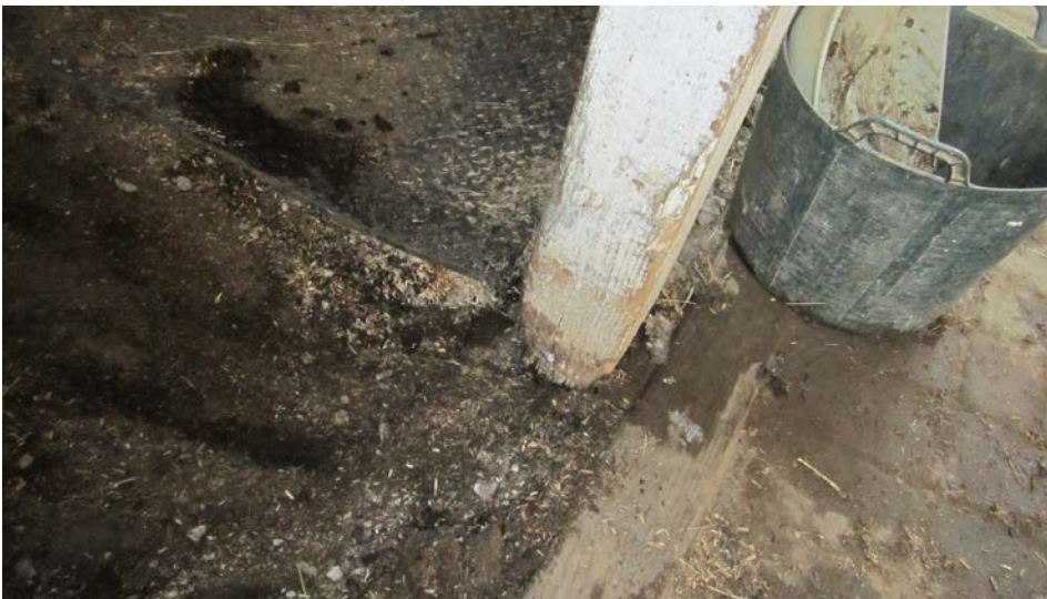
Photo 2 Rotted Interior Post at Stable
